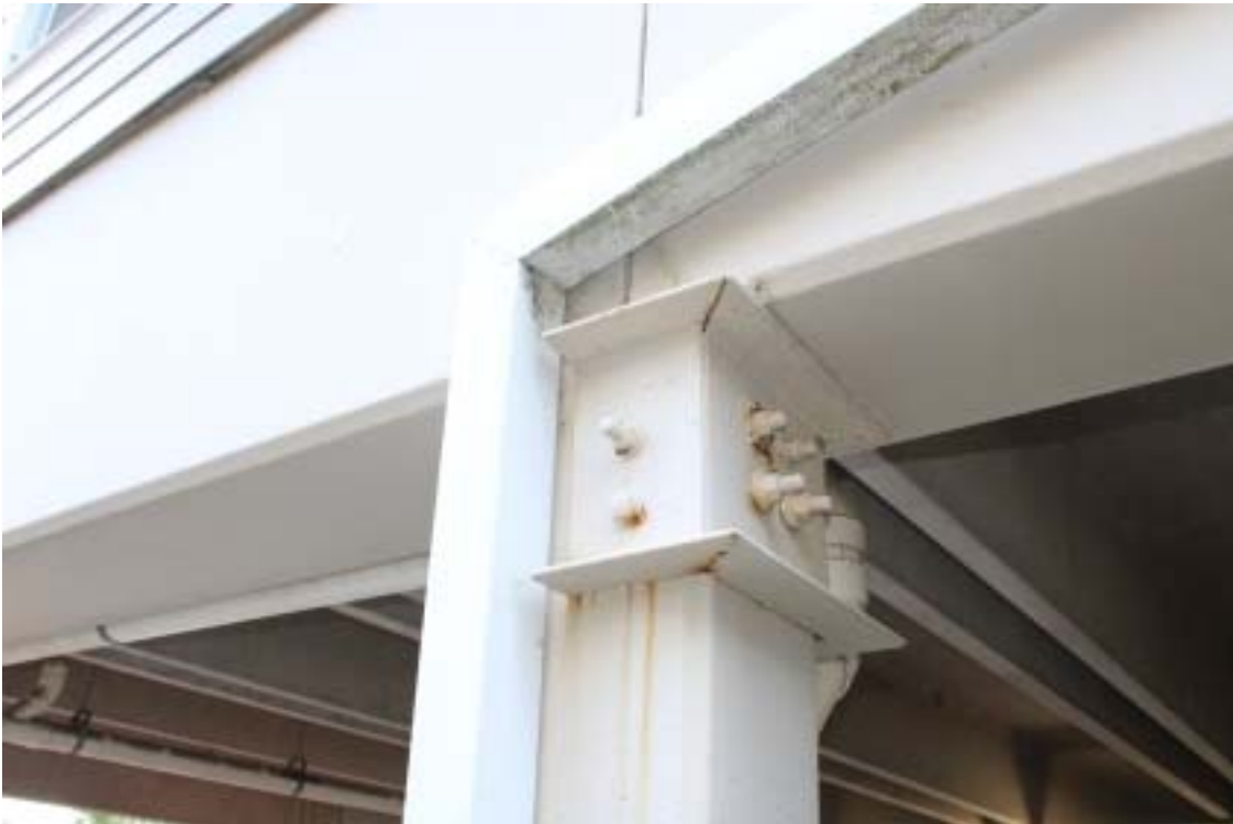
Photograph 40 - Concrete column below precast elements – Note bolted repair and corrosion
