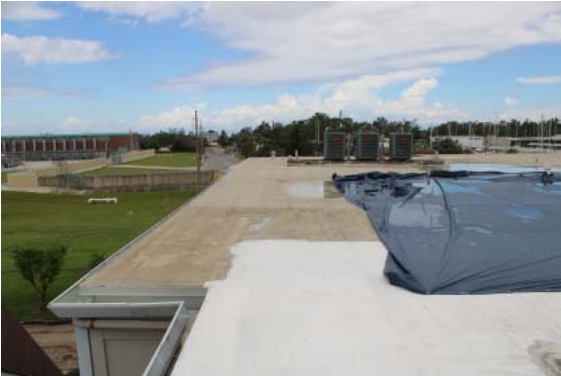
Photograph 19 - Rooftop from west edge – Looking north – Note roof colors and tarp to right
