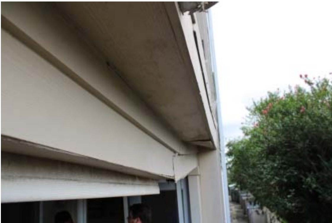
Photograph 72 - West side gallery floor support – Note deflected shape
