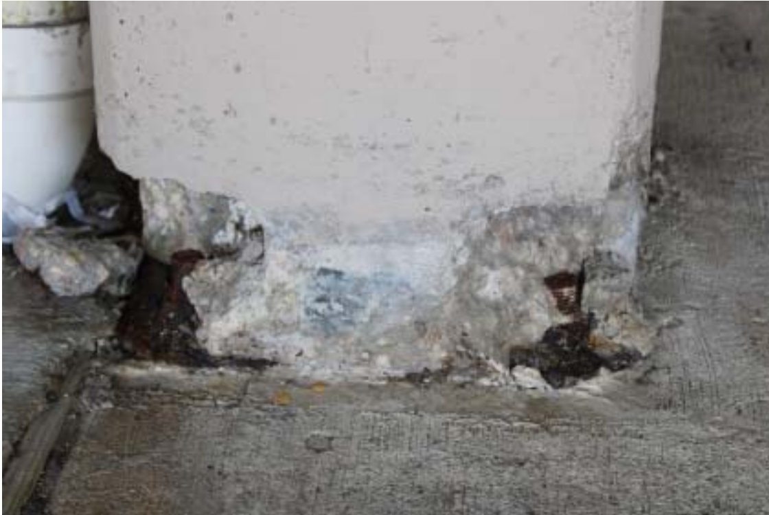
Photograph 57 - Concrete column below precast elements – Note spalled base, anchor bolts, and steel plate
