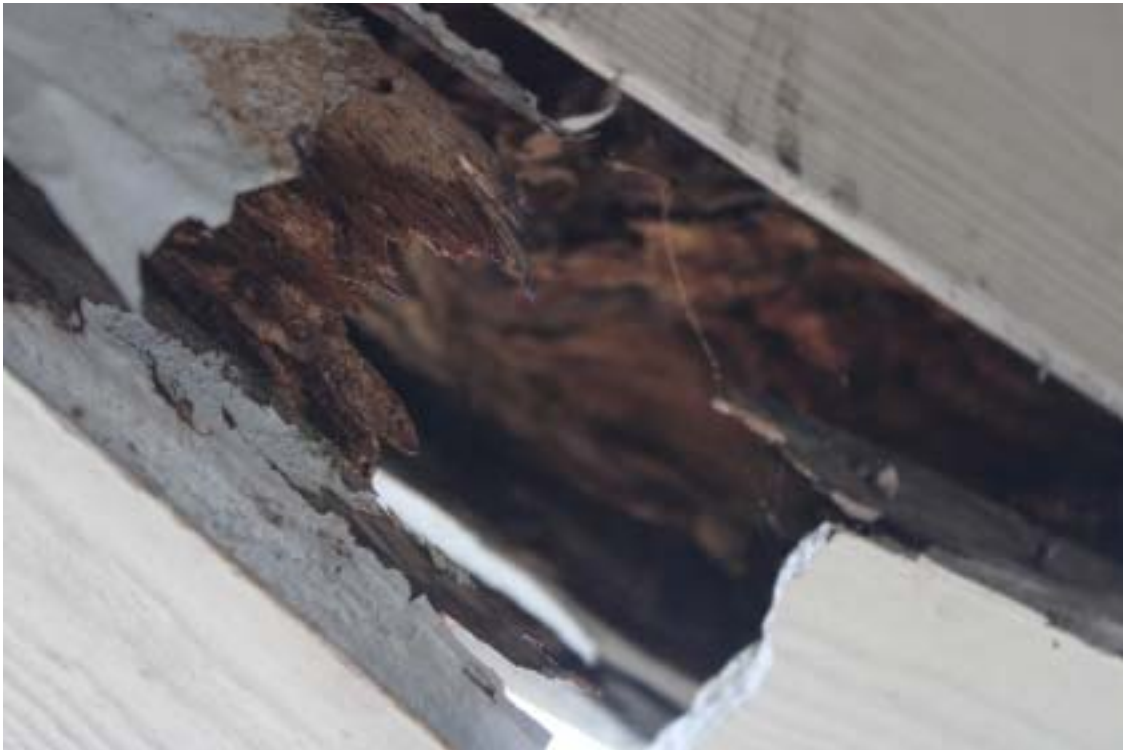
Photograph 76 - West side gallery floor support – Note decayed wood beam
