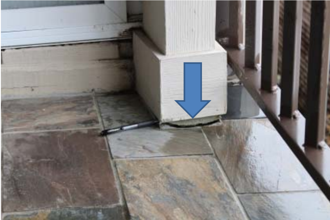
Photograph 69 - West side gallery floor – Note gap between surface and plinth
