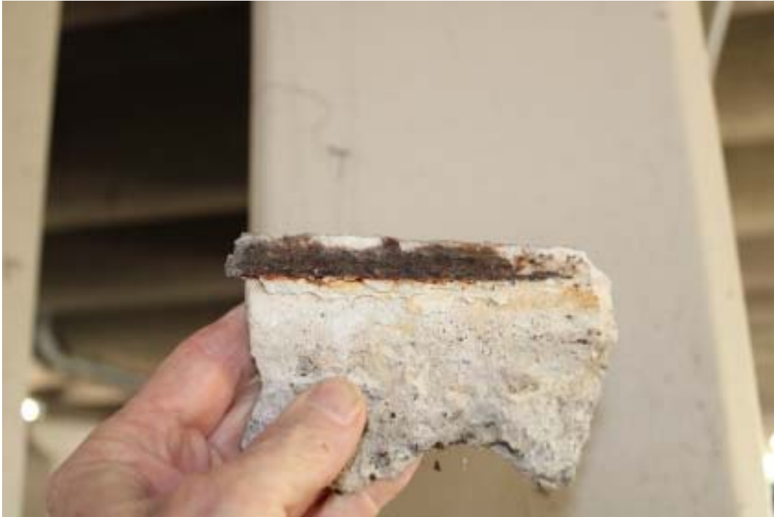
Photograph 53 - Concrete column below precast elements – Note spalled piece from top
