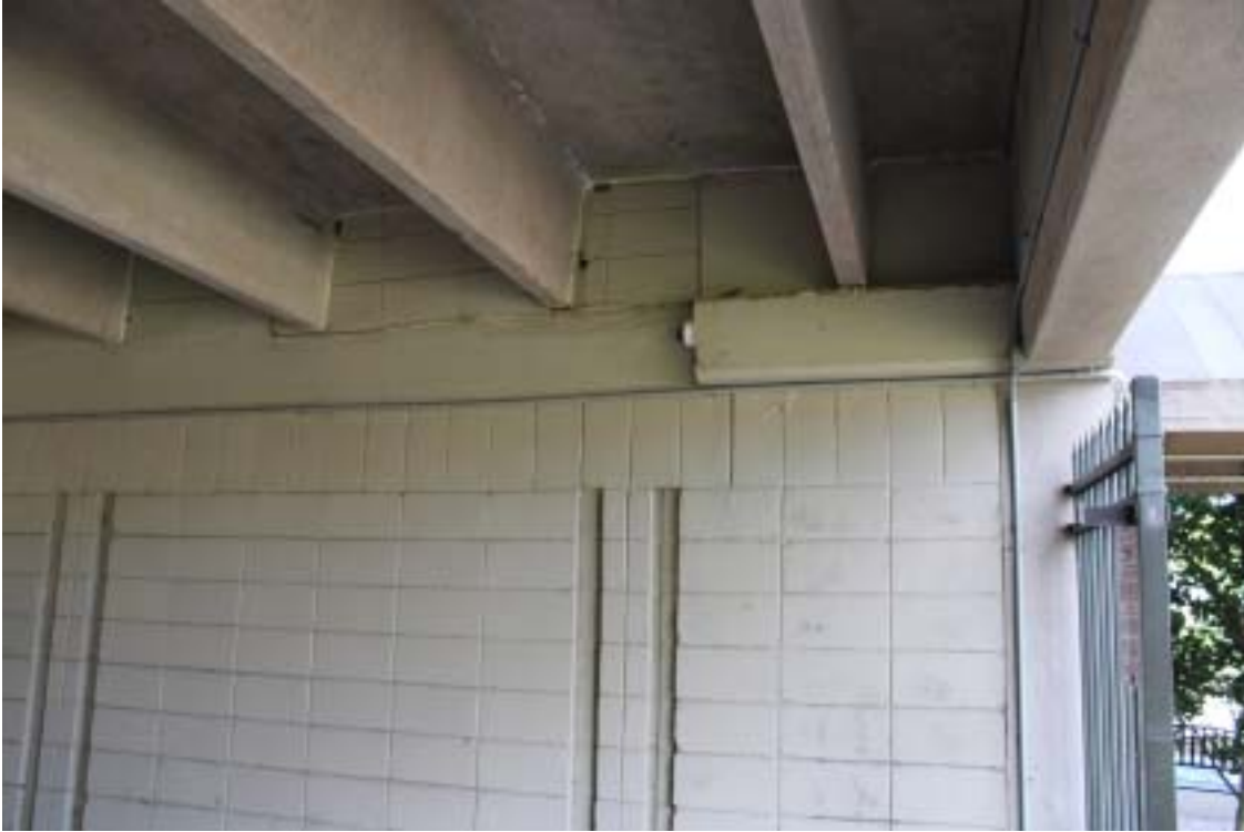
Photograph 35 - Concrete structure above parking level – Wall along office area - Note precast elements
