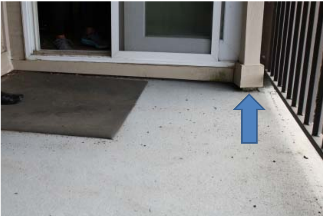
Photograph 68 - West side gallery floor – Note gap between surface and plinth
