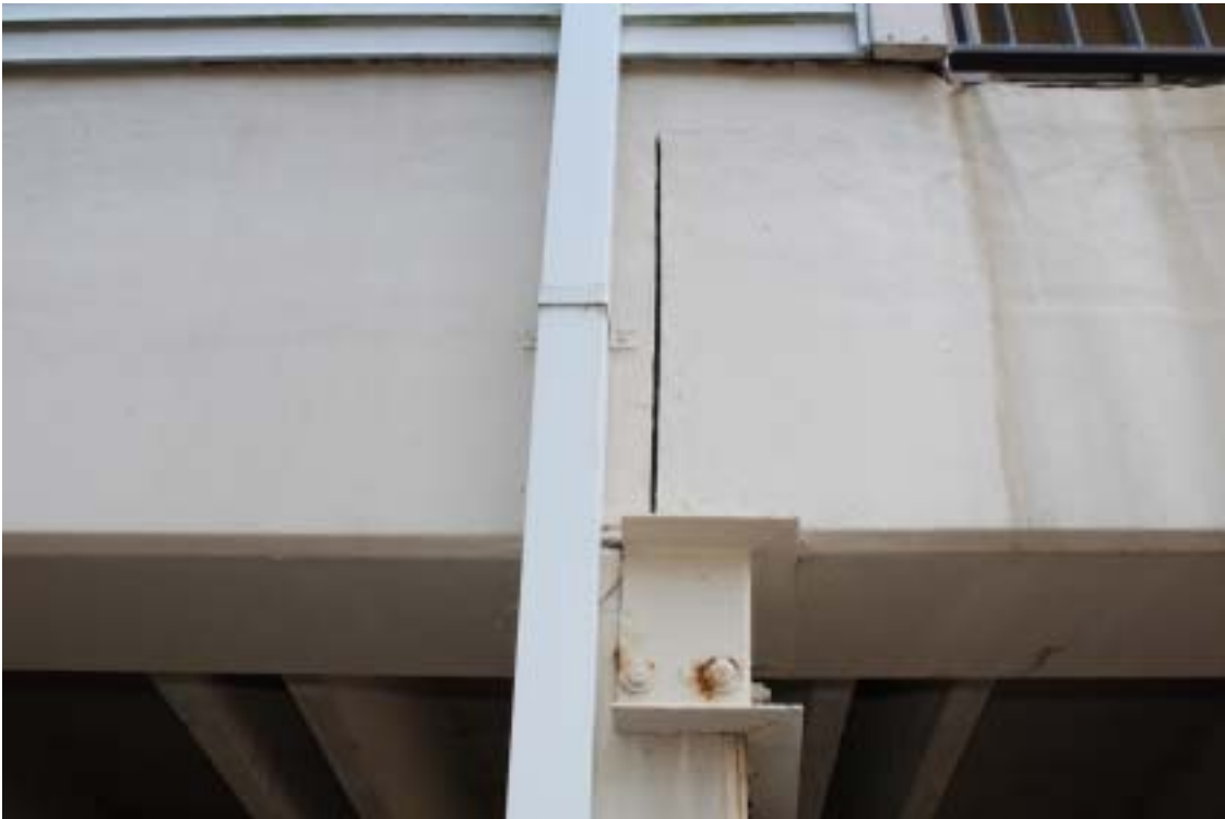
Photograph 46 - Concrete column below precast elements – Note bolted repair
