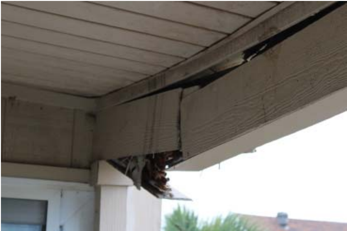
Photograph 74 - West side gallery floor support – Note deflected shape and damaged support beam
