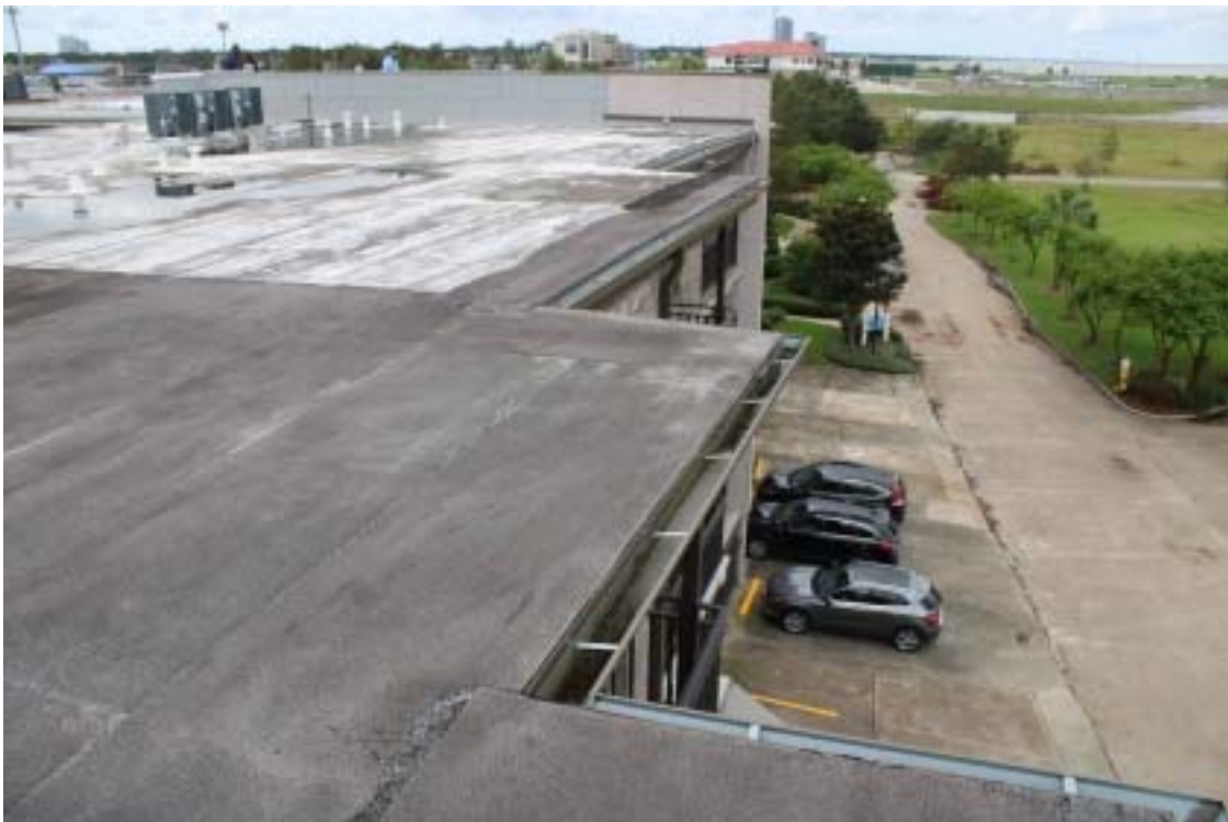
Photograph 16 - Rooftop from northeast corner – Note patched area
