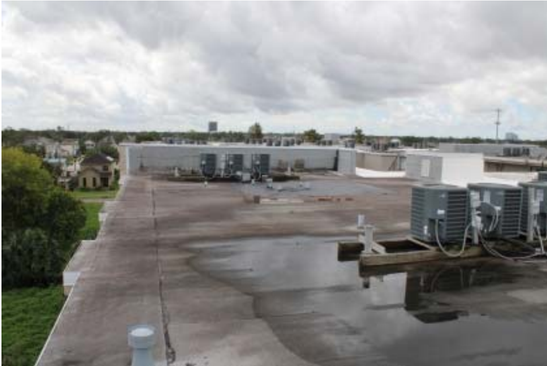
Photograph 15 - Rooftop from northeast corner – Note standing water
