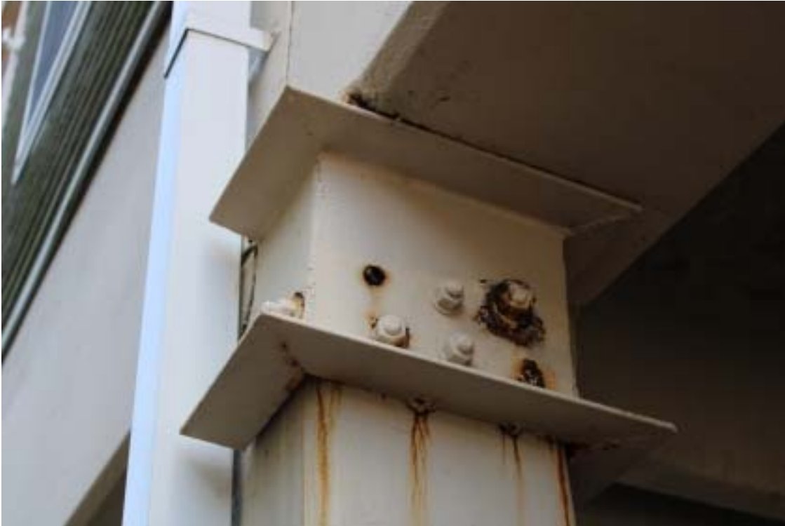
Photograph 47 - Concrete column below precast elements – Note corroded bolted repair
