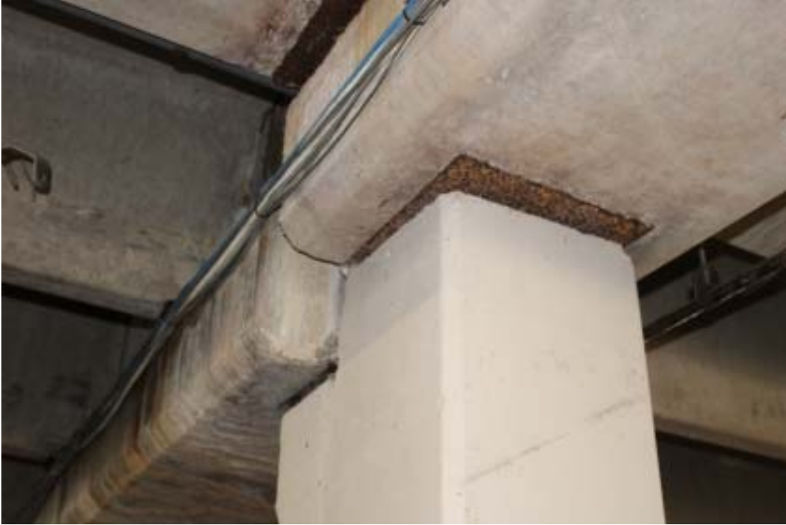
Photograph 37 - Concrete structure above parking level – Note some precast elements were not centered on the bearing plates.
