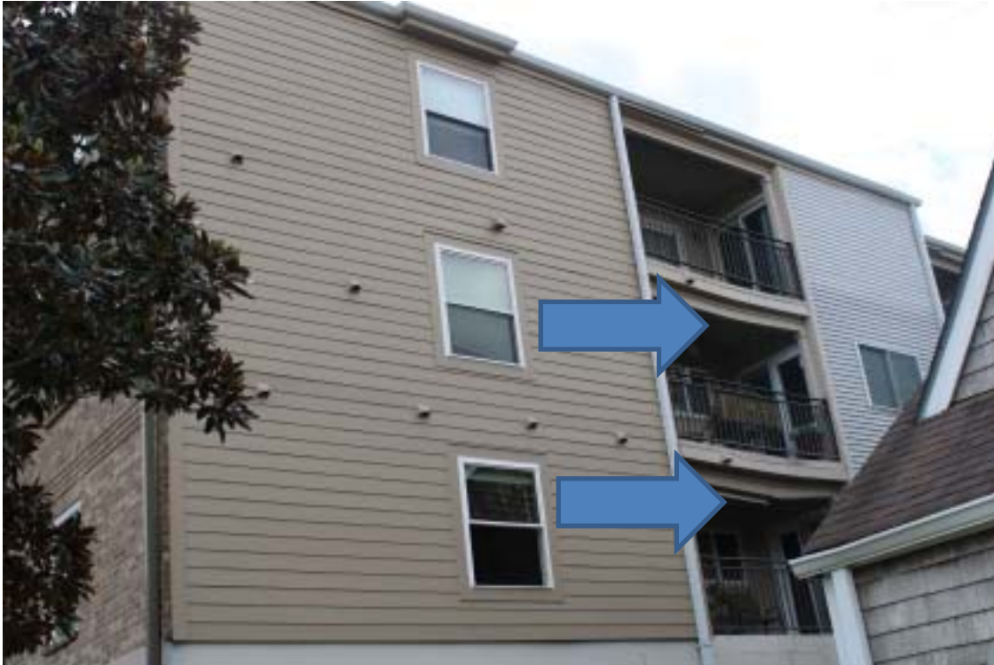
Photograph 3 - Northwest corner of building – Note upper side galleries and deflection indicated
