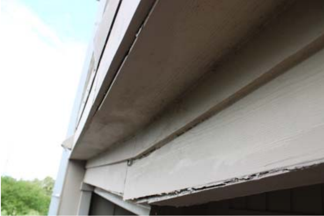
Photograph 75 - West side gallery floor support – Note deflected shape
