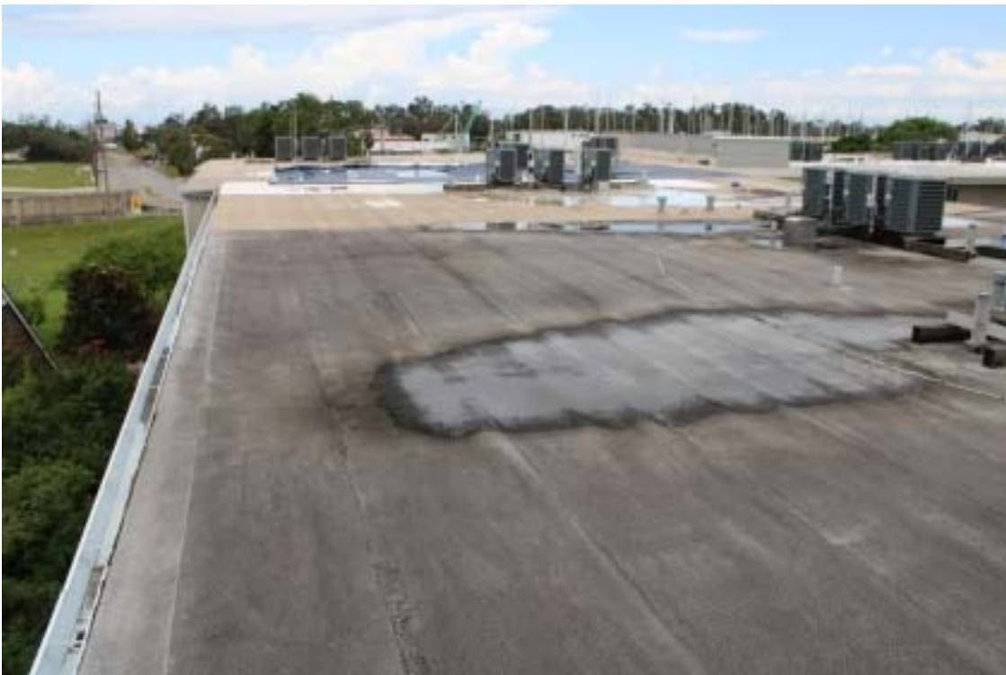
Photograph 20 - Rooftop from west edge – Looking north – Note roof colors and ponding
