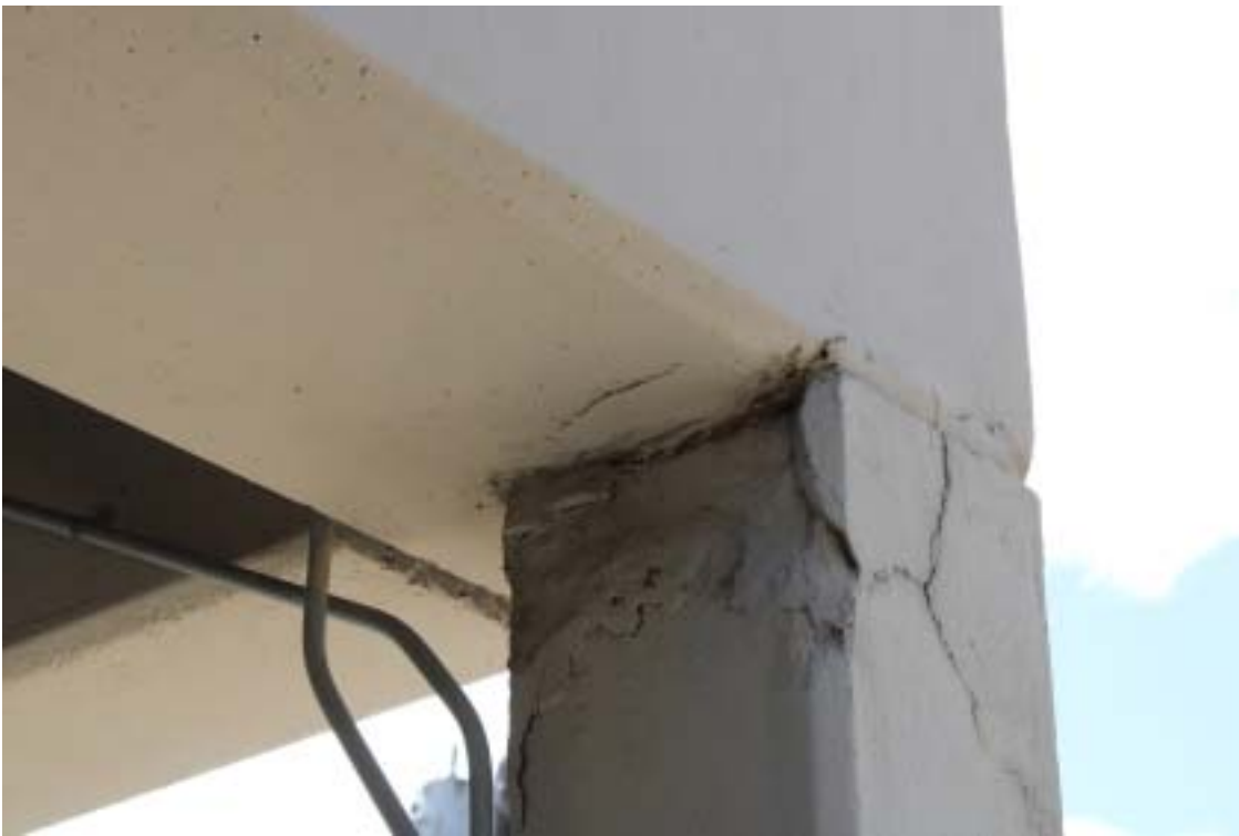
Photograph 48 - Concrete column below precast elements – Note spalling at top and coating over the spalled pieces
