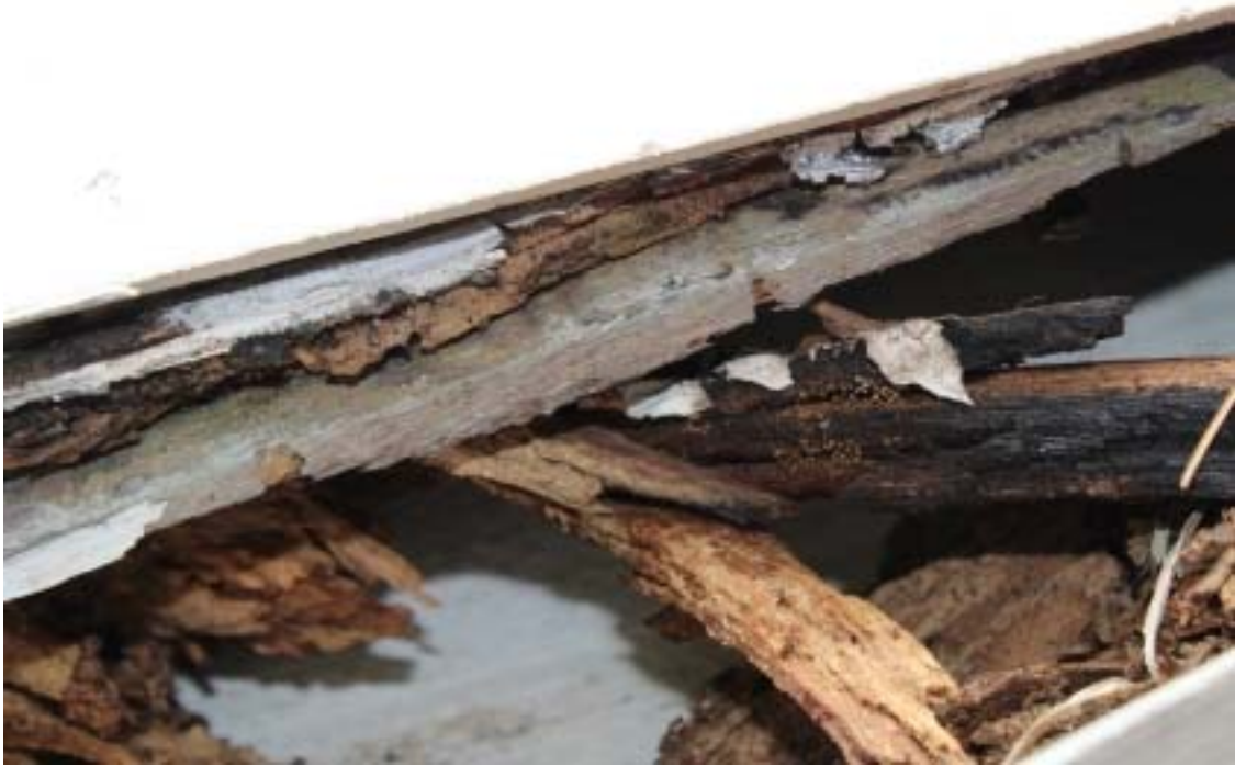
Photograph 77 - West side gallery floor support – Note decayed wood beam
