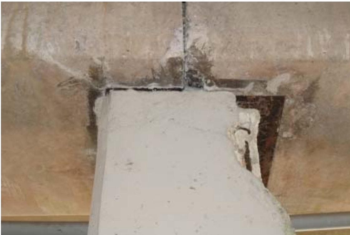
Photograph 54 - Concrete column below precast elements – Note spalled top and steel plate
