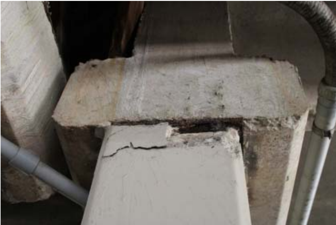
Photograph 52 - Concrete column below precast elements – Note spalling at top
