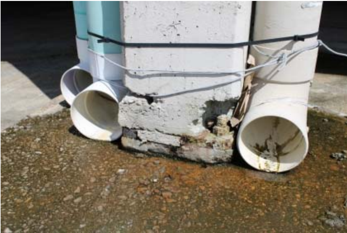
Photograph 56 - Concrete column below precast elements – Note spalled base, anchor bolt, and steel plate
