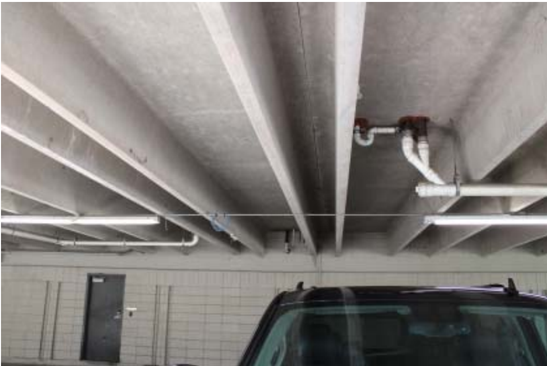
Photograph 34 - Concrete structure above parking level – Wall along office area - Note precast elements
