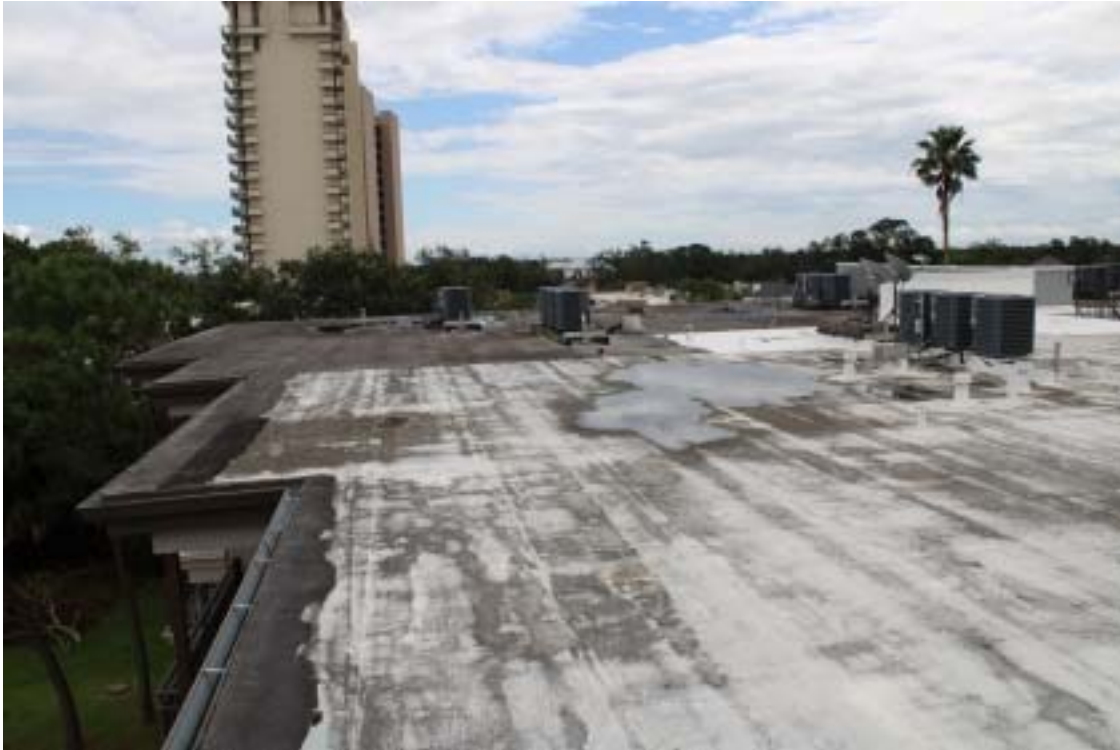
Photograph 17 - Rooftop from north edge – Note light-colored patched area
