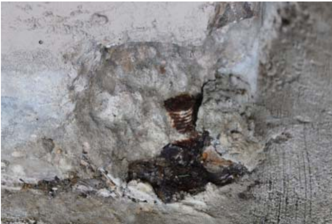
Photograph 58 - Concrete column below precast elements – Note spalled base, anchor bolt, and steel plate
