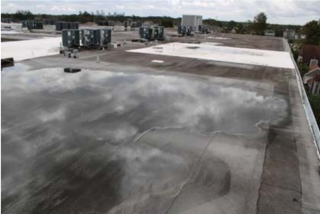
Photograph 23 - Rooftop from west edge – Looking south – Note varying roof colors and ponding
