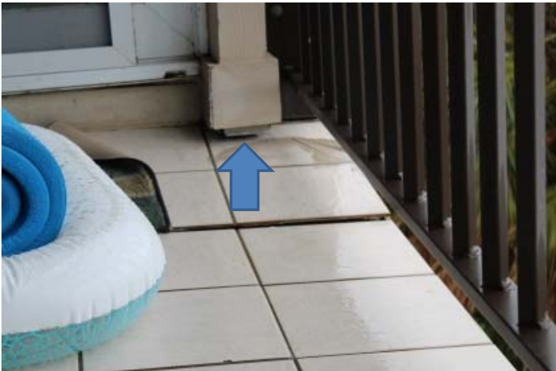
Photograph 70 - West side gallery floor – Note gap between surface and plinth
