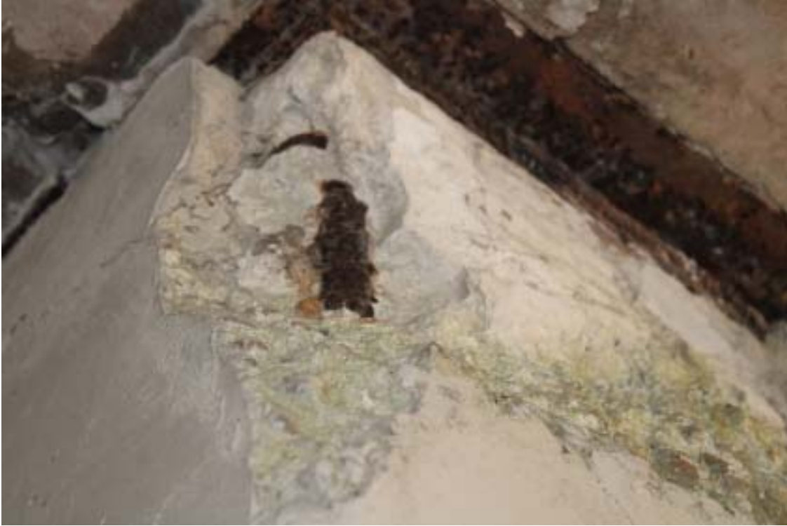
Photograph 55 - Concrete column below precast elements – Note spalled top and steel plate
