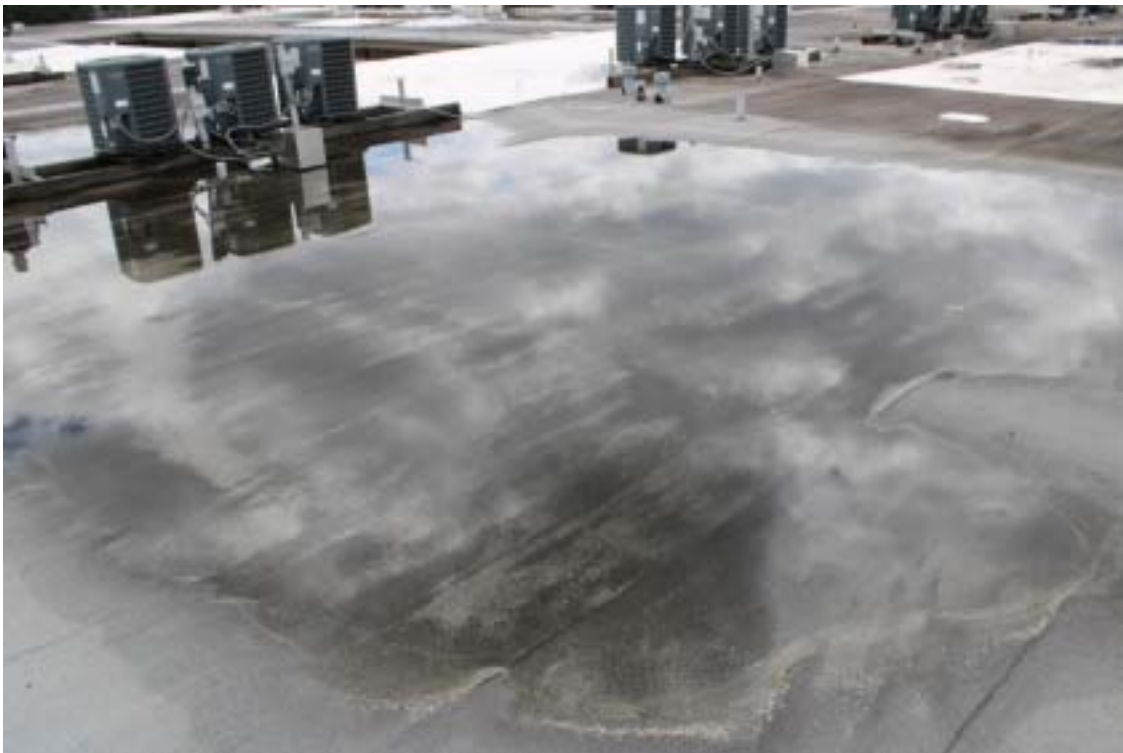
Photograph 24 - Rooftop from west edge – Looking southeast – Note ponding
