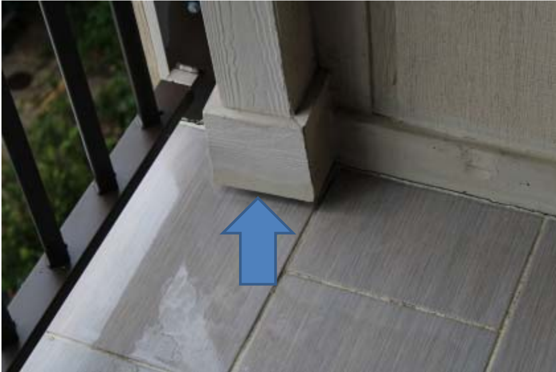
Photograph 71 - West side gallery floor – Note gap between surface and plinth
