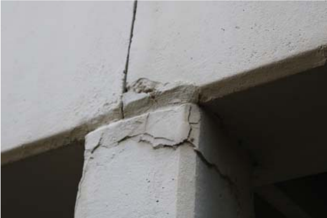
Photograph 41 - Concrete column below precast elements – Note spalling at top
