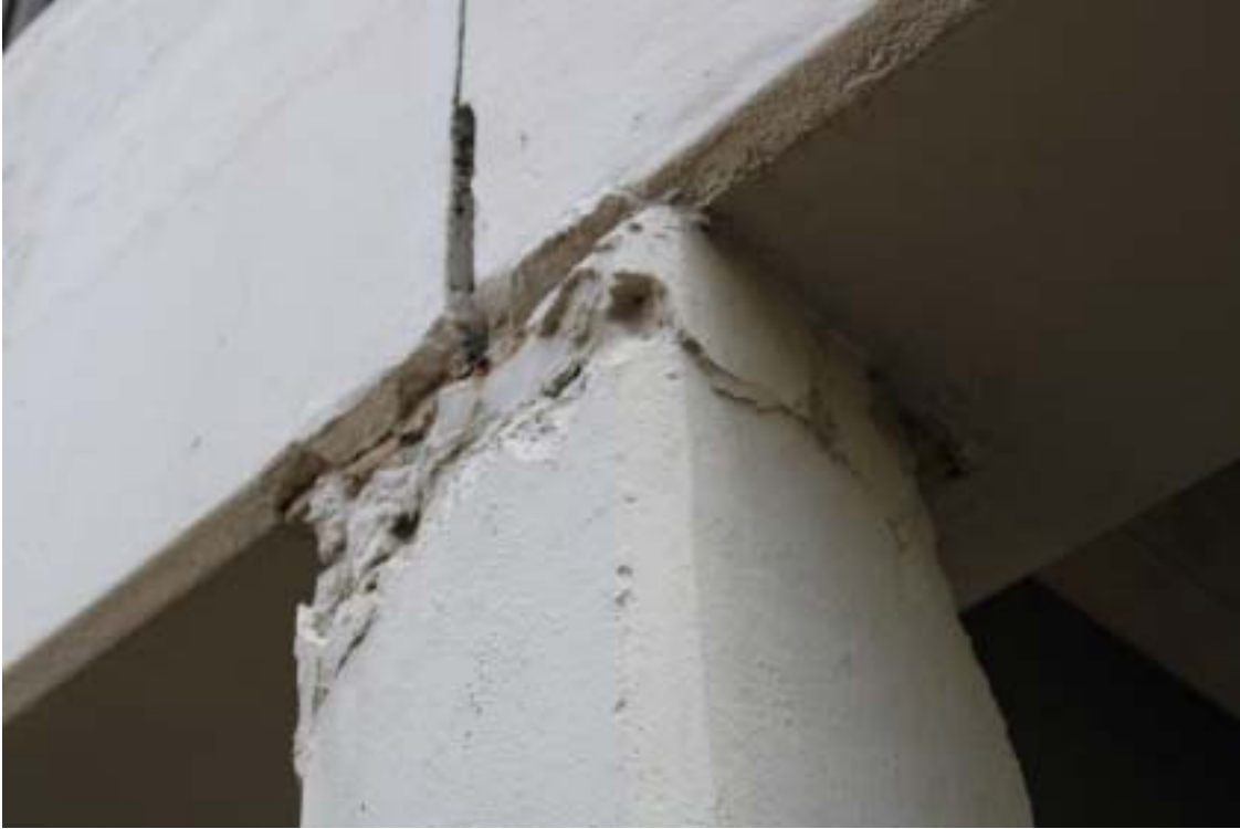
Photograph 45 - Concrete column below precast elements – Note spalling at top
