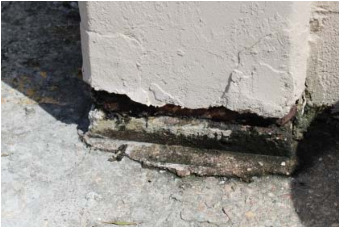
Photograph 50 - Concrete column below precast elements – Note section loss cracking at base
