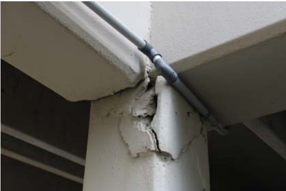
Photograph 42 - Concrete column below precast elements – Note spalling at top and coating over the spalled pieces
