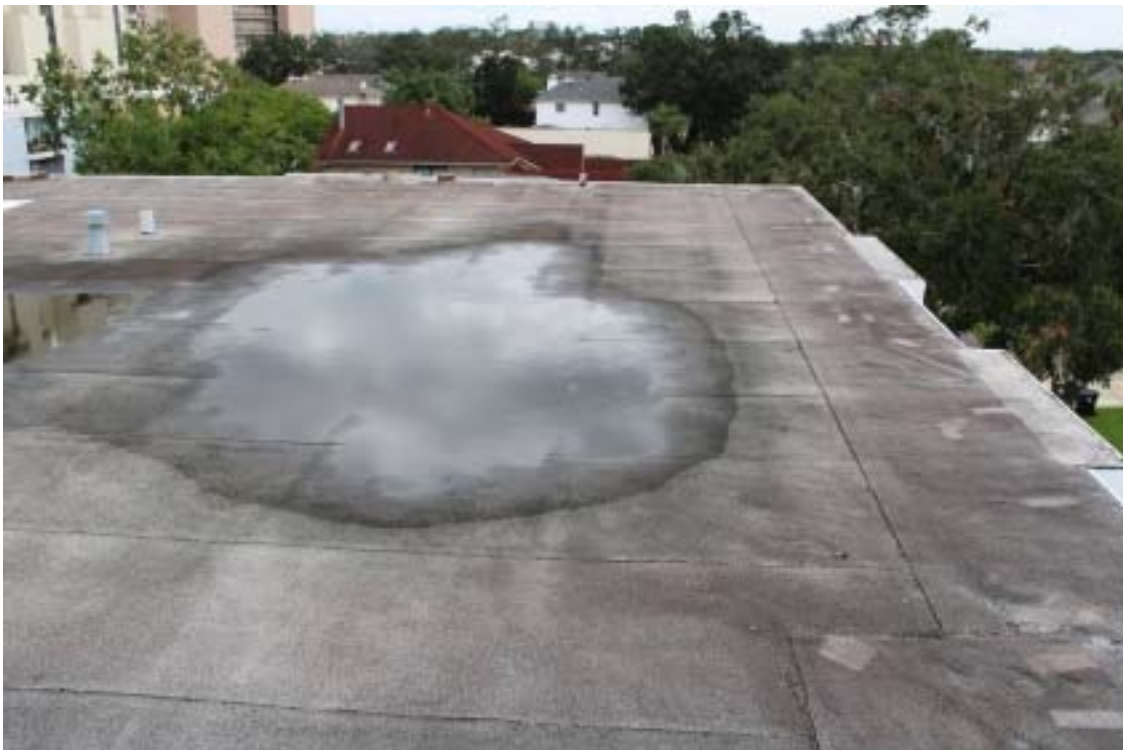
Photograph 28 - Rooftop from south edge – Looking east – Note ponding
