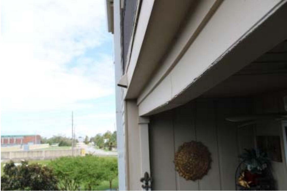
Photograph 73 - West side gallery floor support – Note deflected shape
