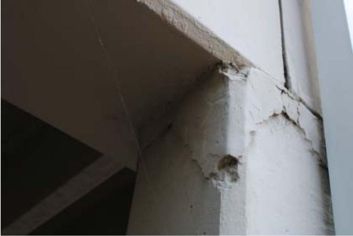
Photograph 43 - Concrete column below precast elements – Note spalling at top and coating over the spalled pieces
