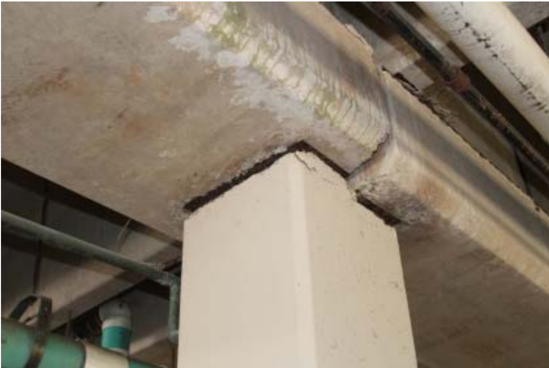
Photograph 38 - Concrete structure above parking level – Note off-center precast elements
