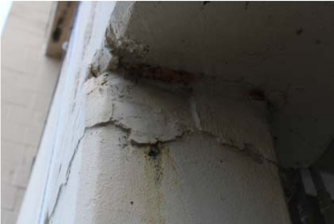
Photograph 44 - Concrete column below precast elements – Note spalling at top
