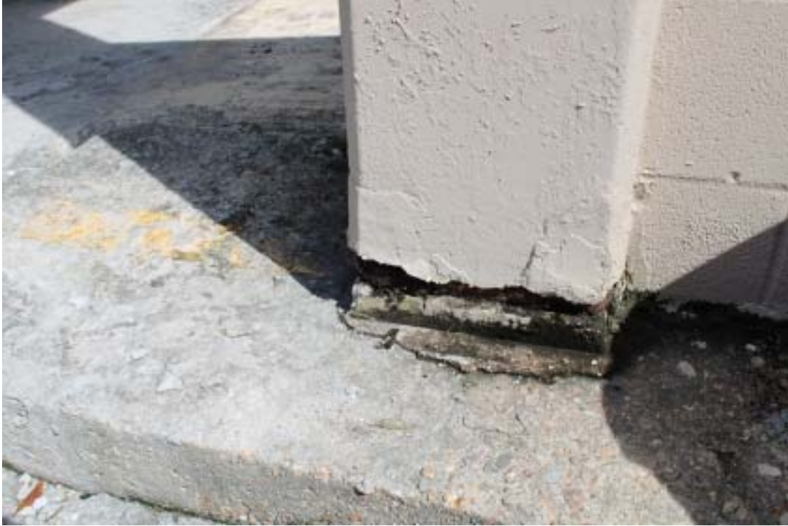
Photograph 49 - Concrete column below precast elements – Note section loss at base
