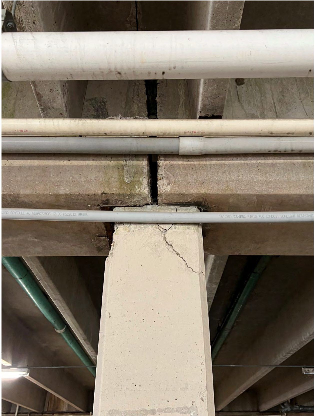
Photo #13 – Column 2 of 2 where shoring is required. 12 th column from N-E corner at 1 st interior bay.
