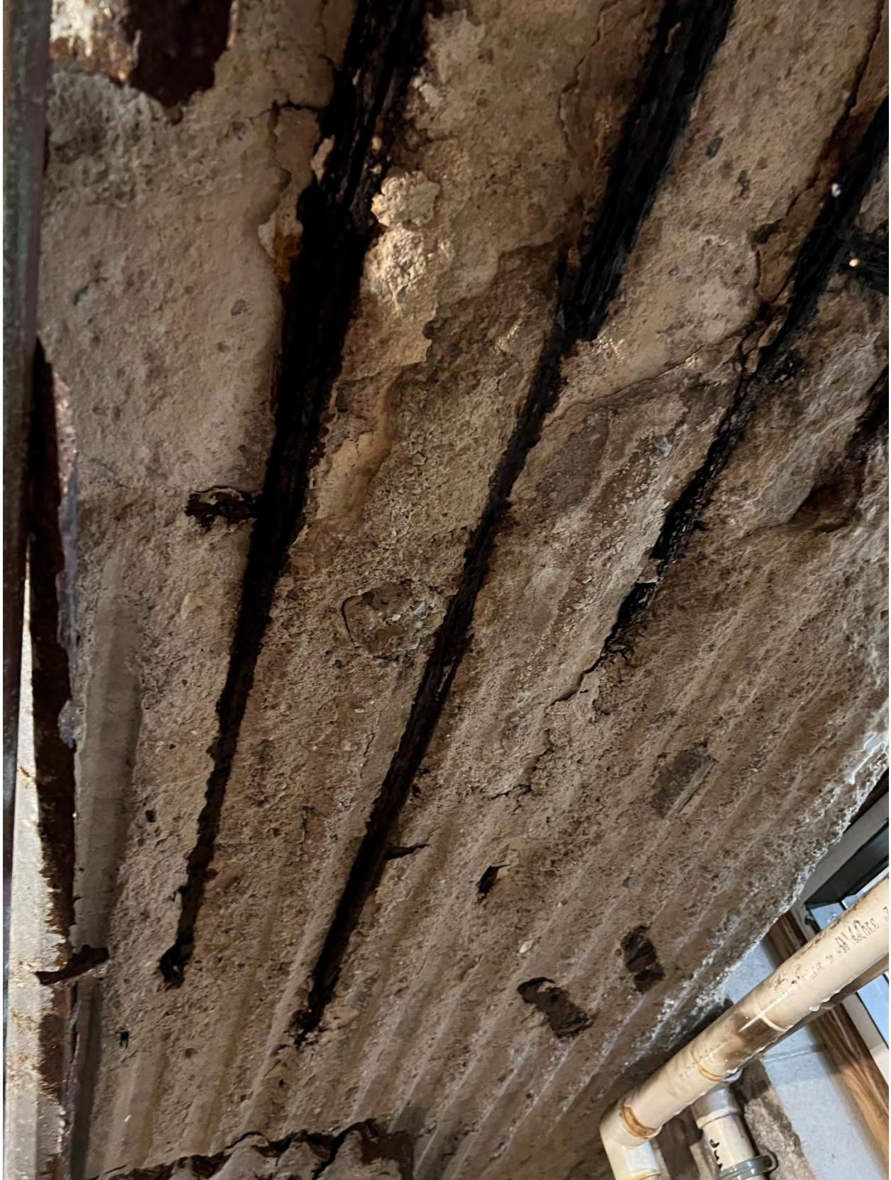
Photo #18 – Close-up view of corroded reinforcing showing signs of significant loss of section
