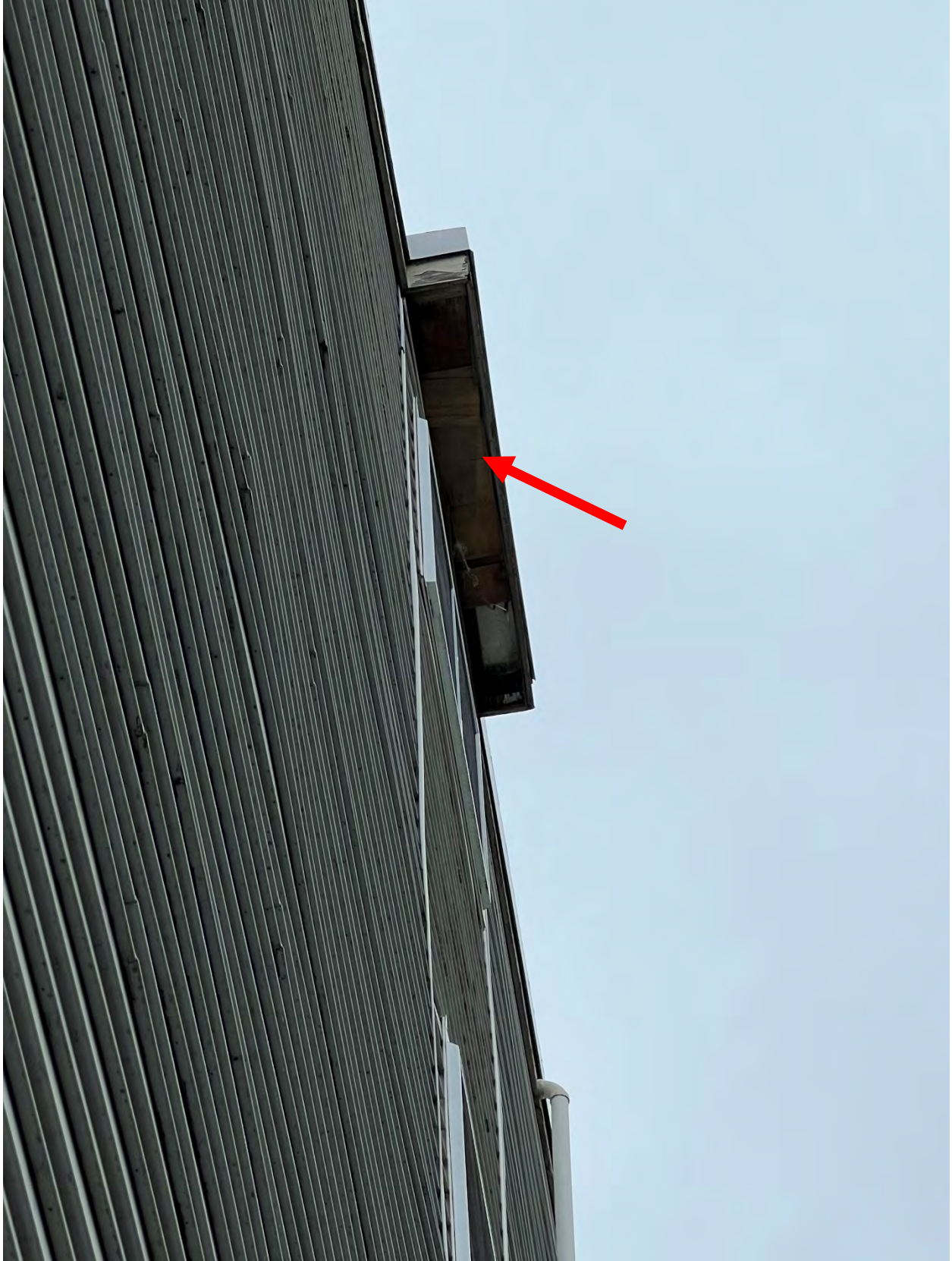
Photo #8 – View of wind related damage to roof soffits at east wall.
