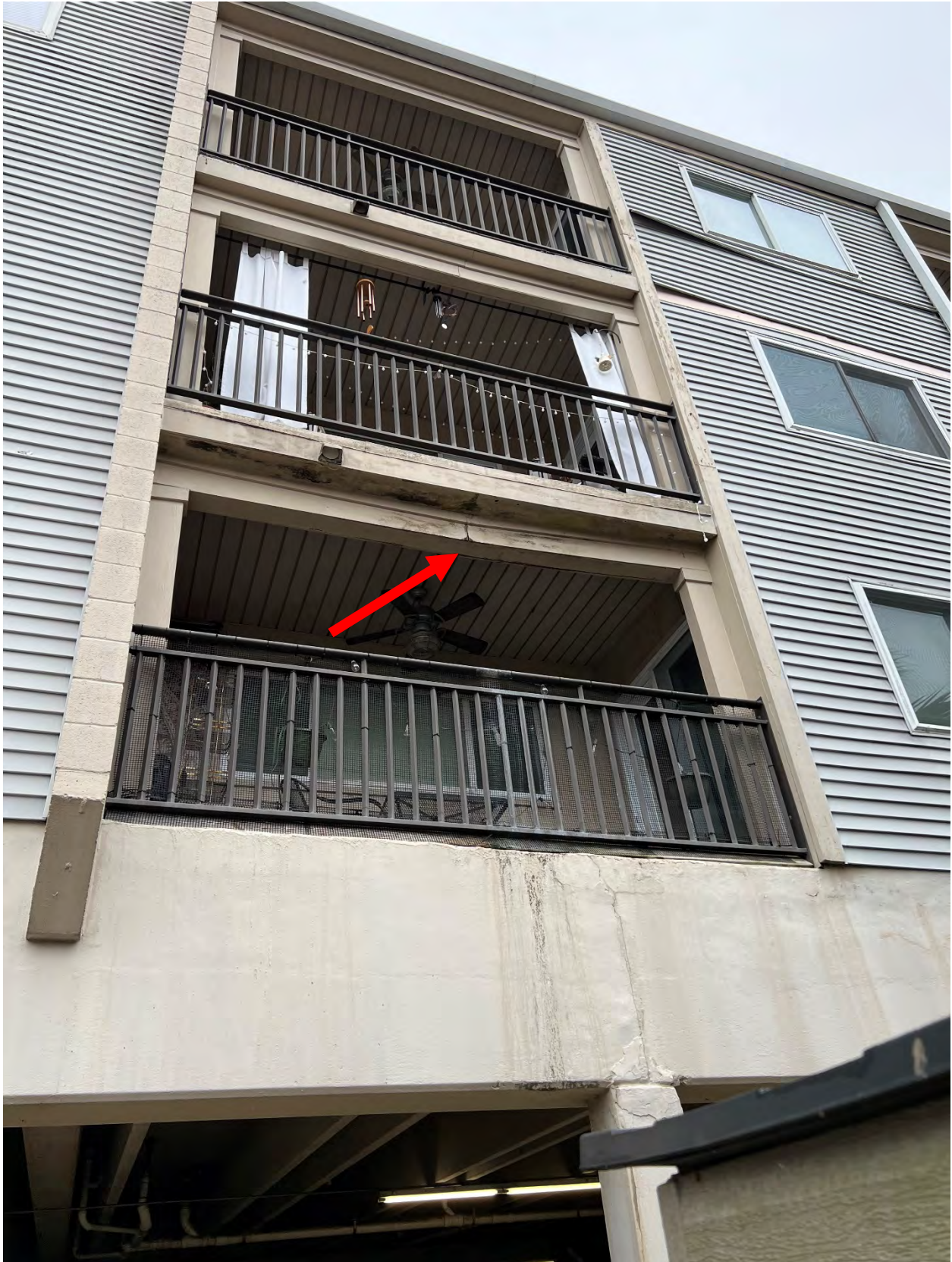
Photo #2 – View of partial balcony failure exhibiting noticeable deflection and water damage.
