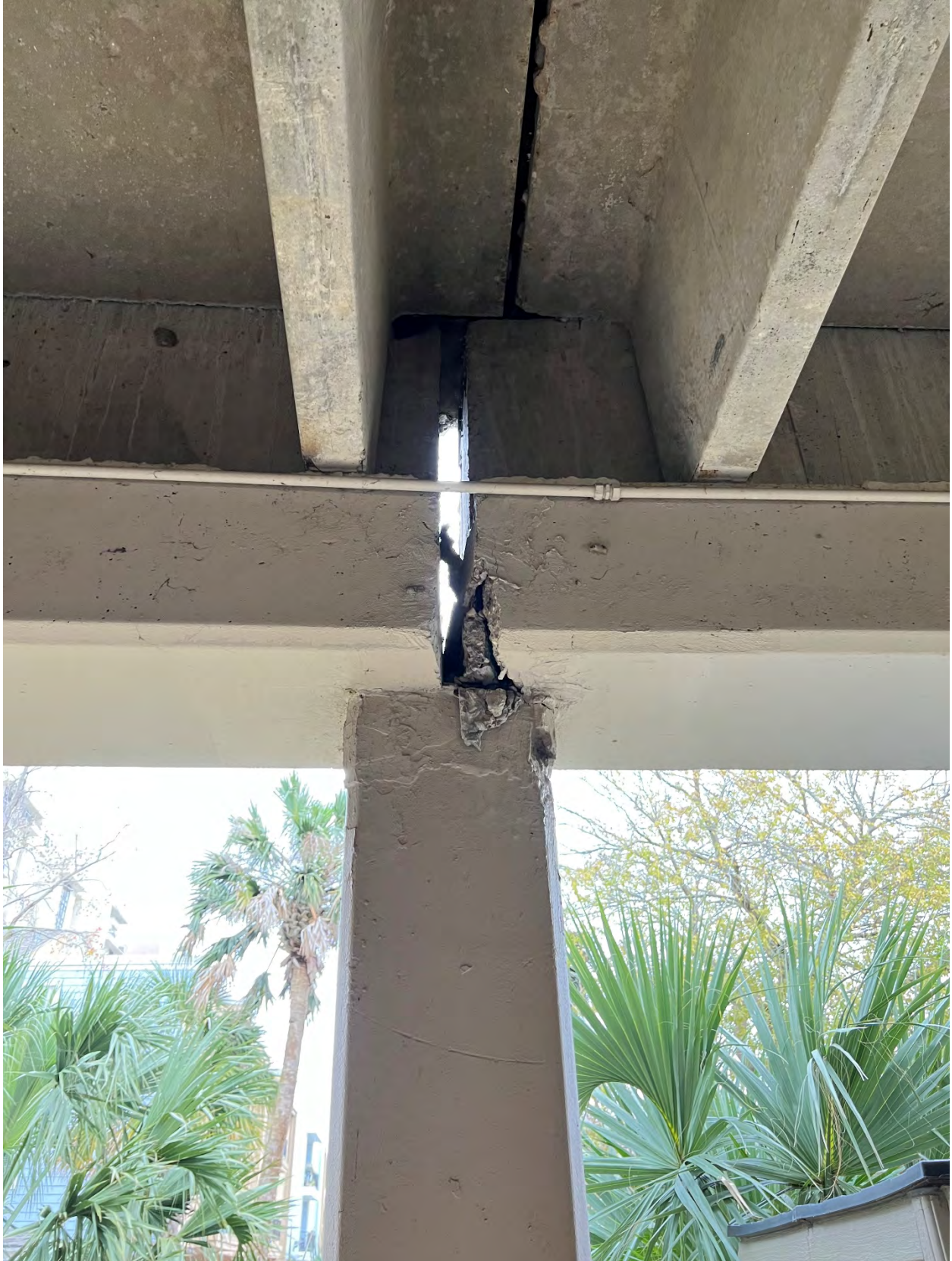
Photo #11 – Column 1 of 2 where shoring is required. 10 th column from N-E corner.
