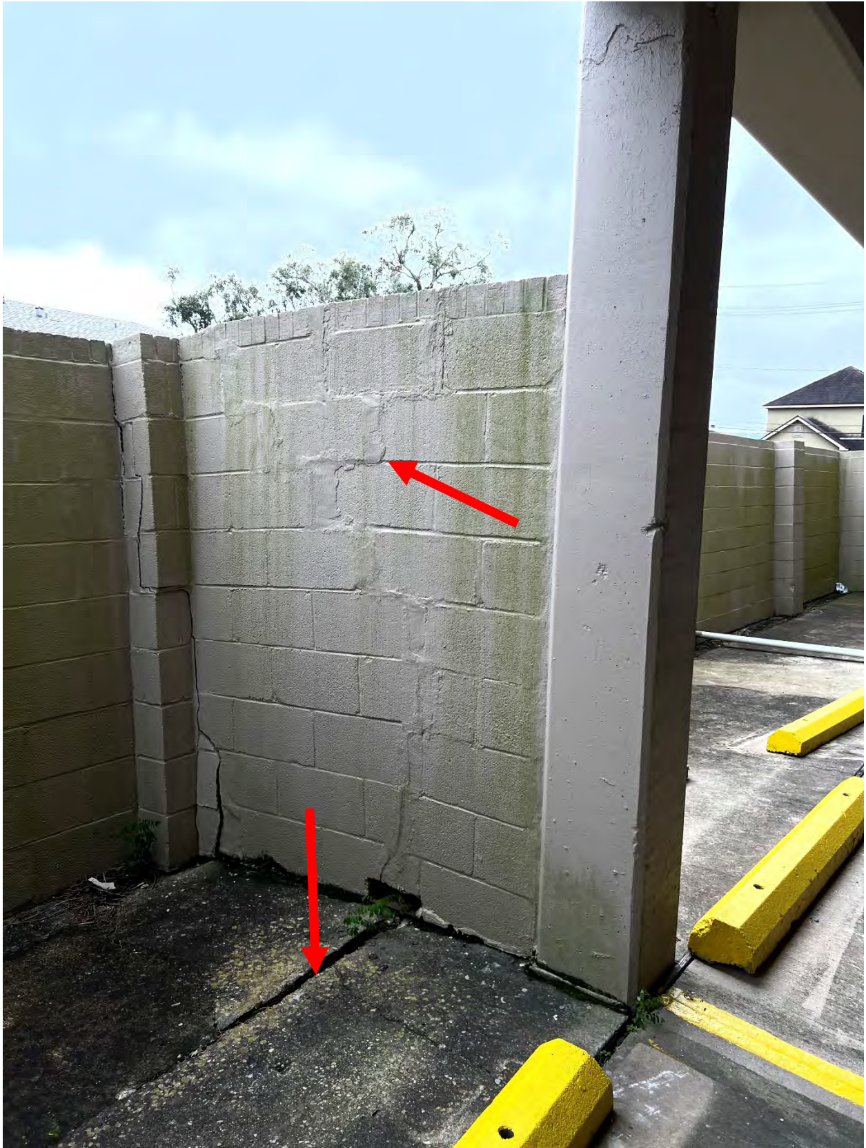
Photo #10 – View of CMU enclosure wall exhibiting settlement issues.
