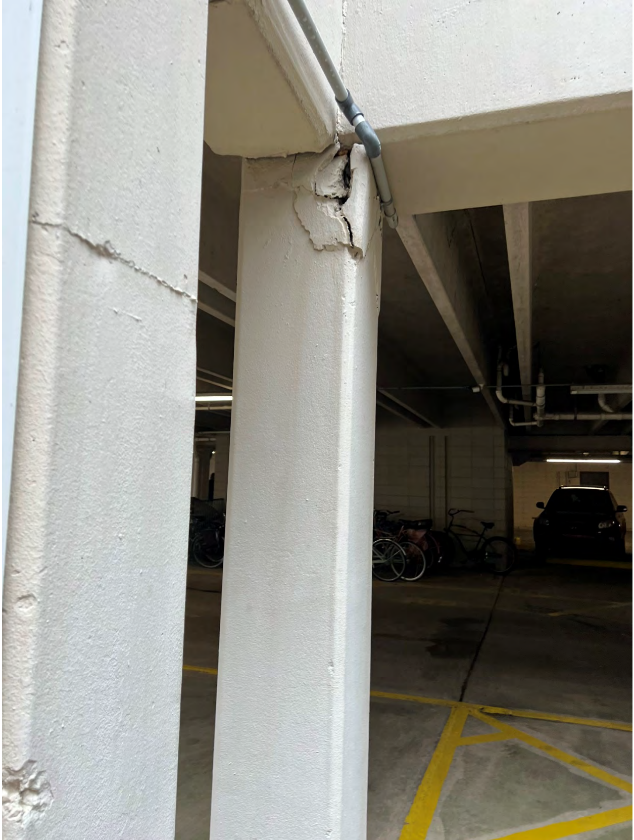
Photo #3 – View of typical top of column concrete spalling.
