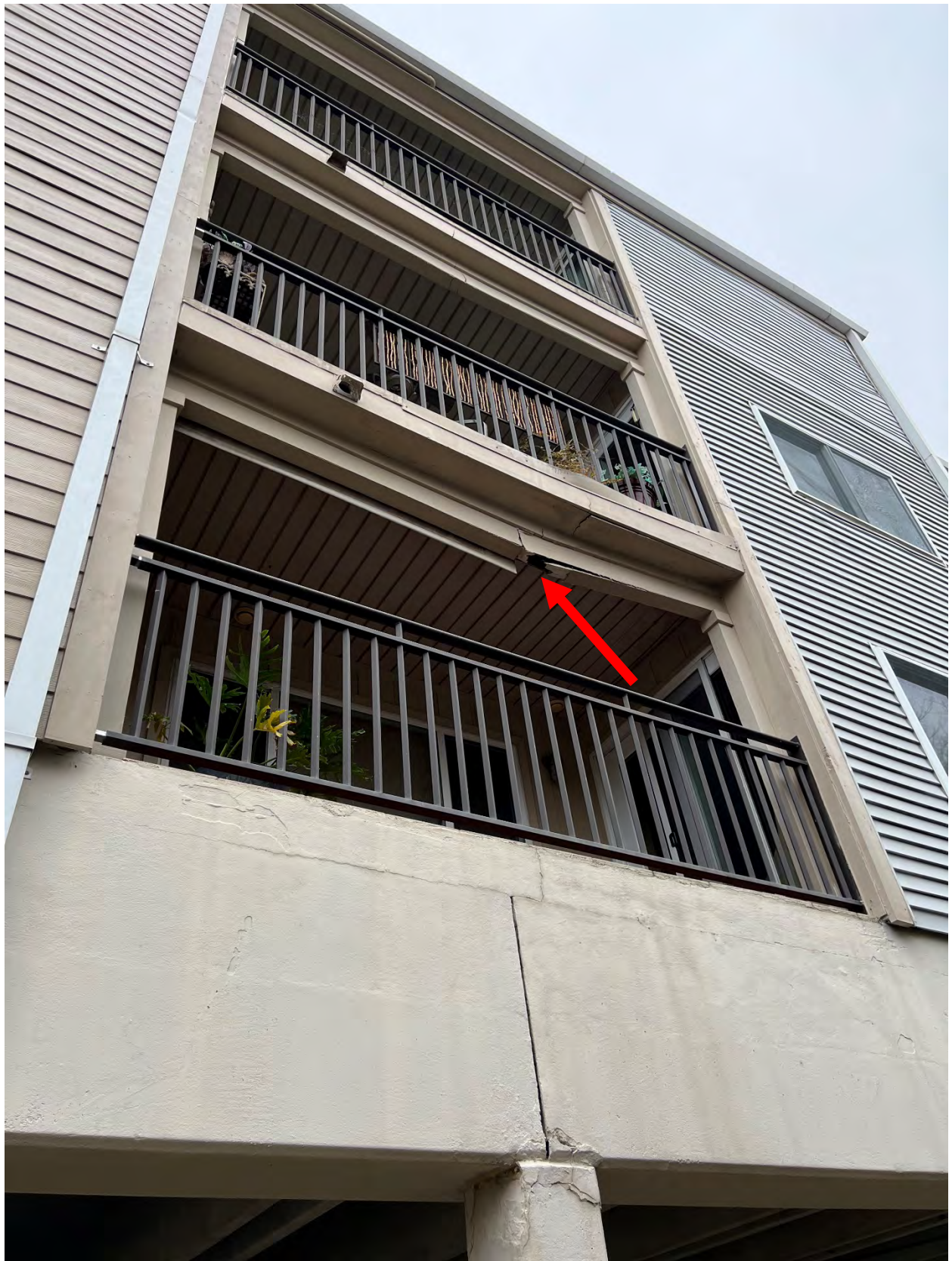
Photo #1 – View of partial balcony failure exhibiting noticeable deflection and water damage.
