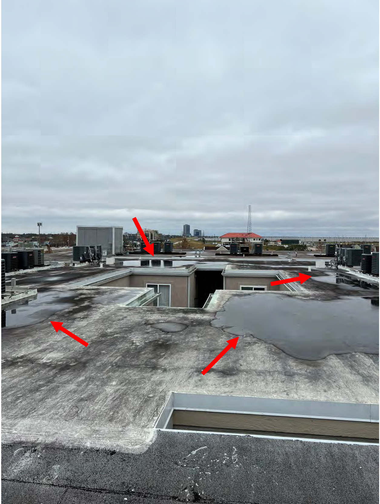
Photo #19 – View of typical ponding at roof.
