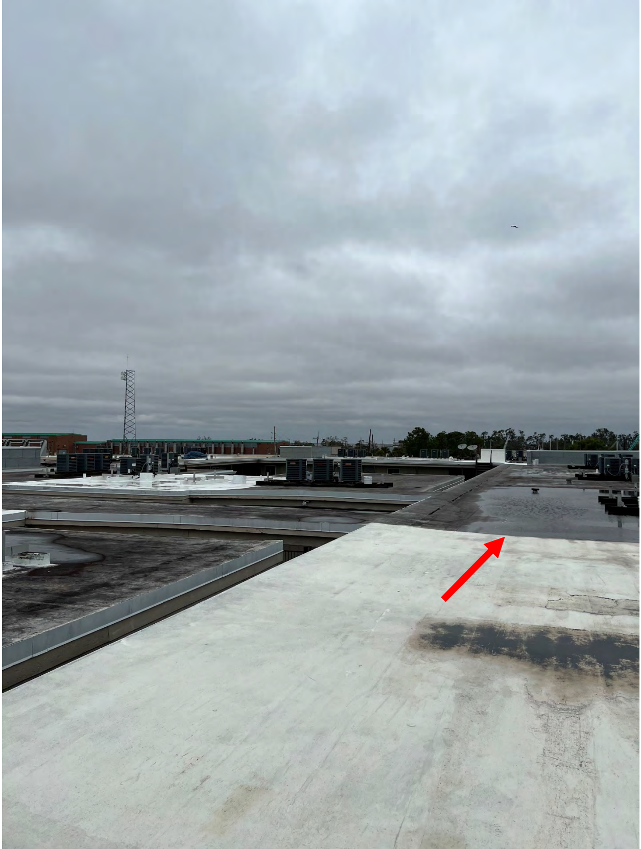
Photo #20 – View of typical ponding at roof.
