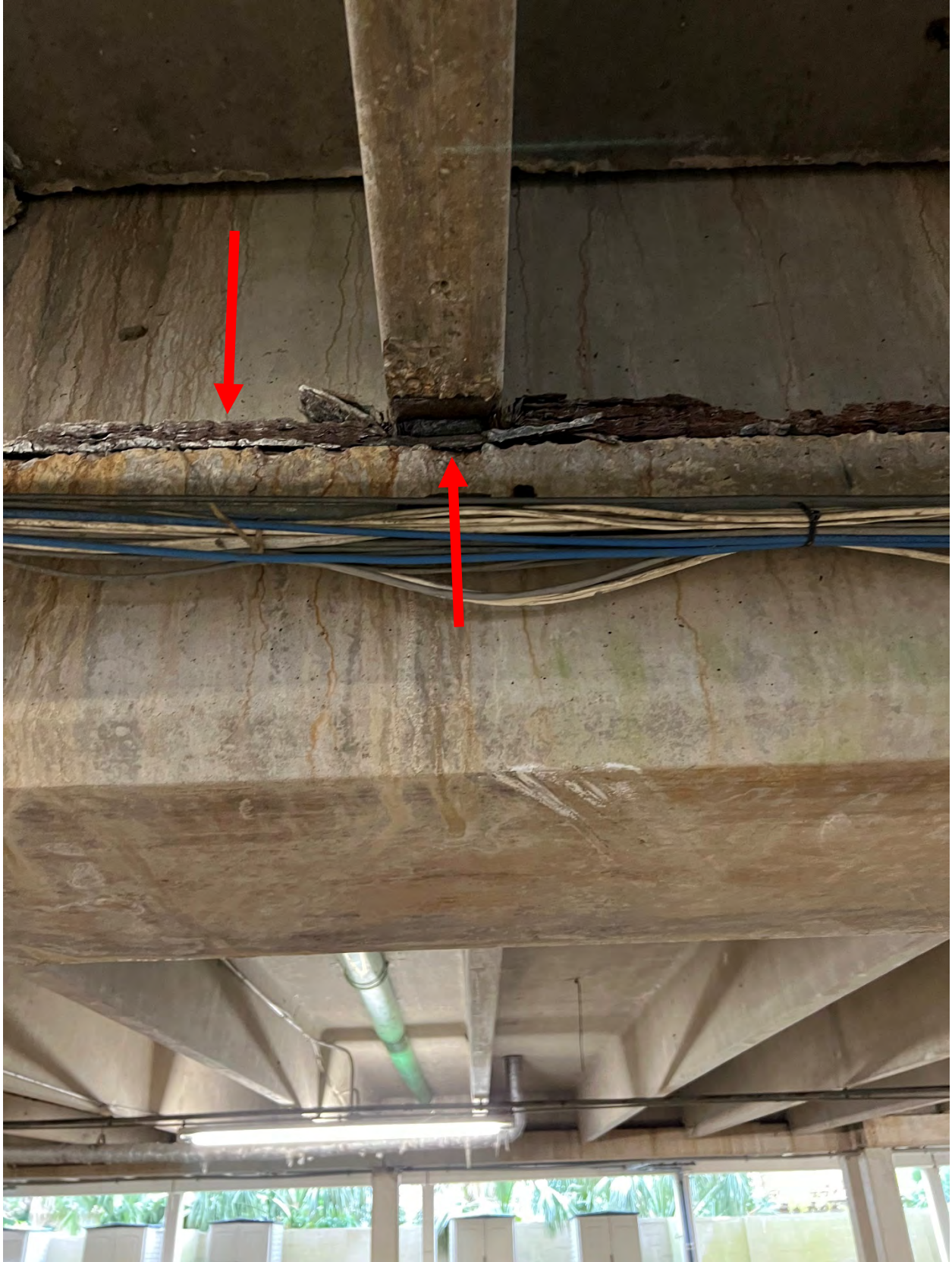
Photo #15 – View of extreme corrosion at double Tee steel bearing angle.
