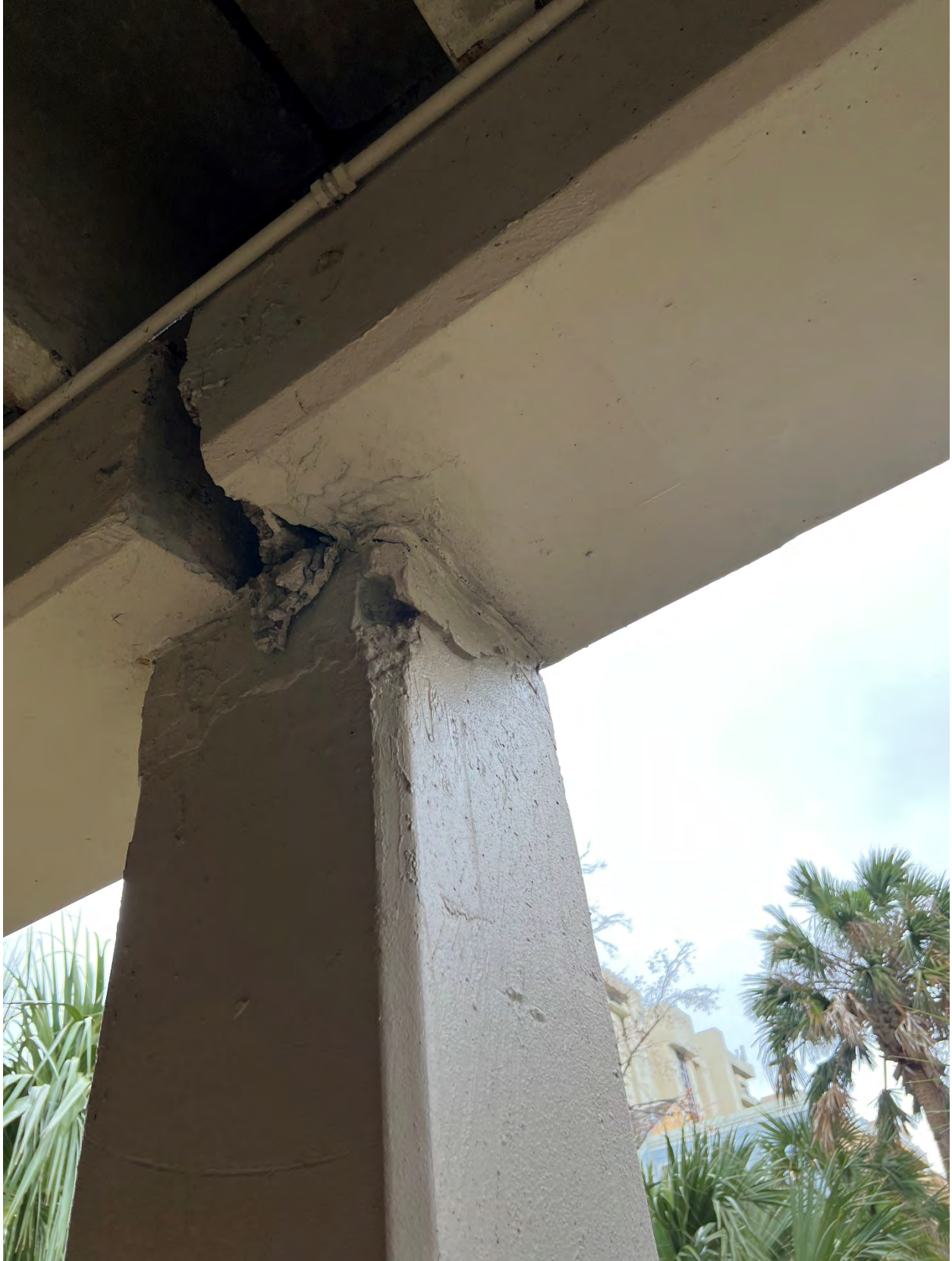
Photo #12 – Close up view of column in photo #11 showing minimal beam support.
