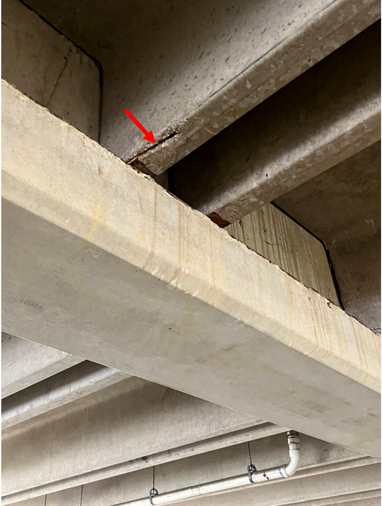
Photo #14 – View of typical corrosion at precast double Tee ends.
