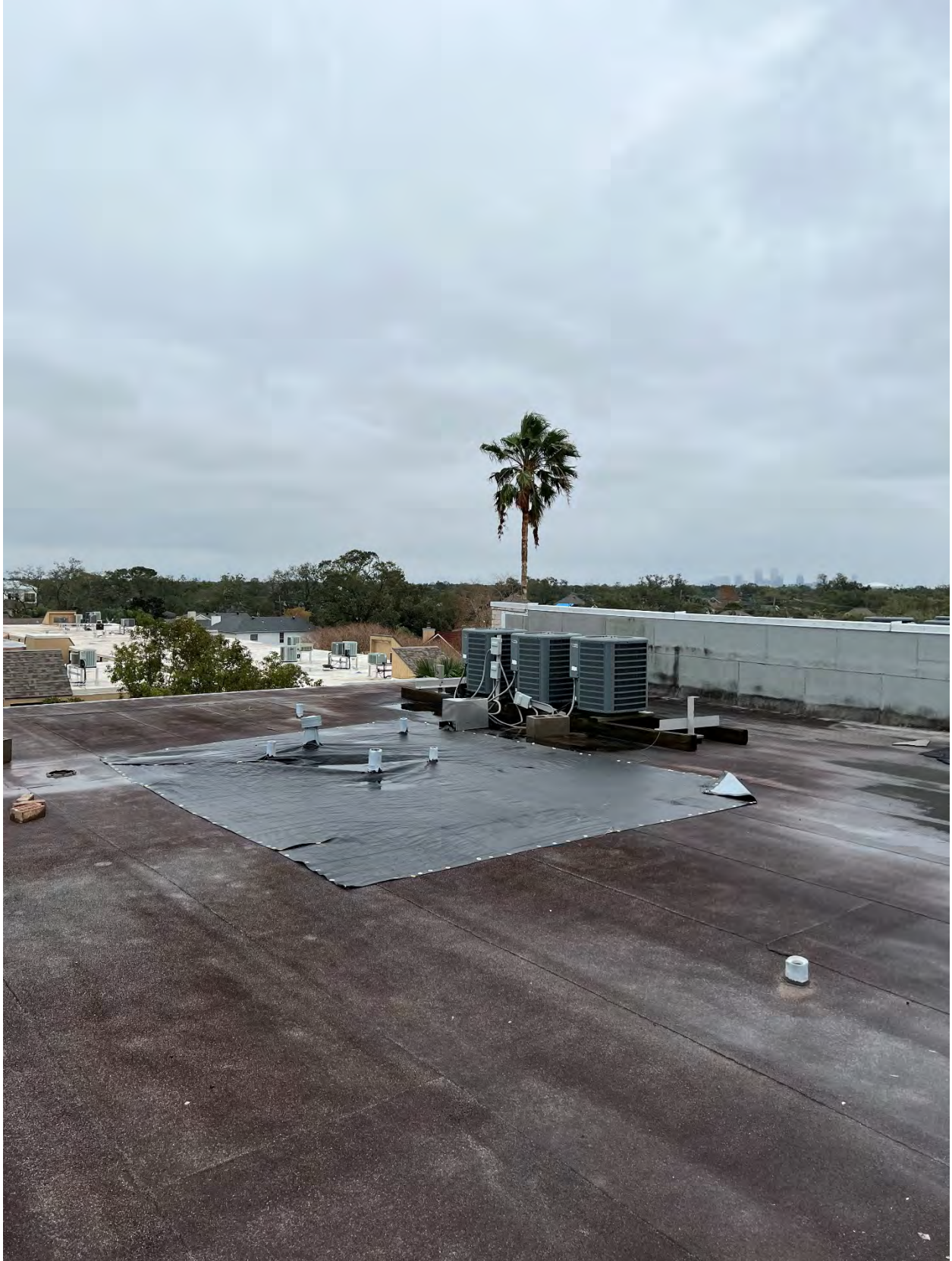
Photo #21 – View of tarped roof area presumably the result of hurricane related wind damage.
