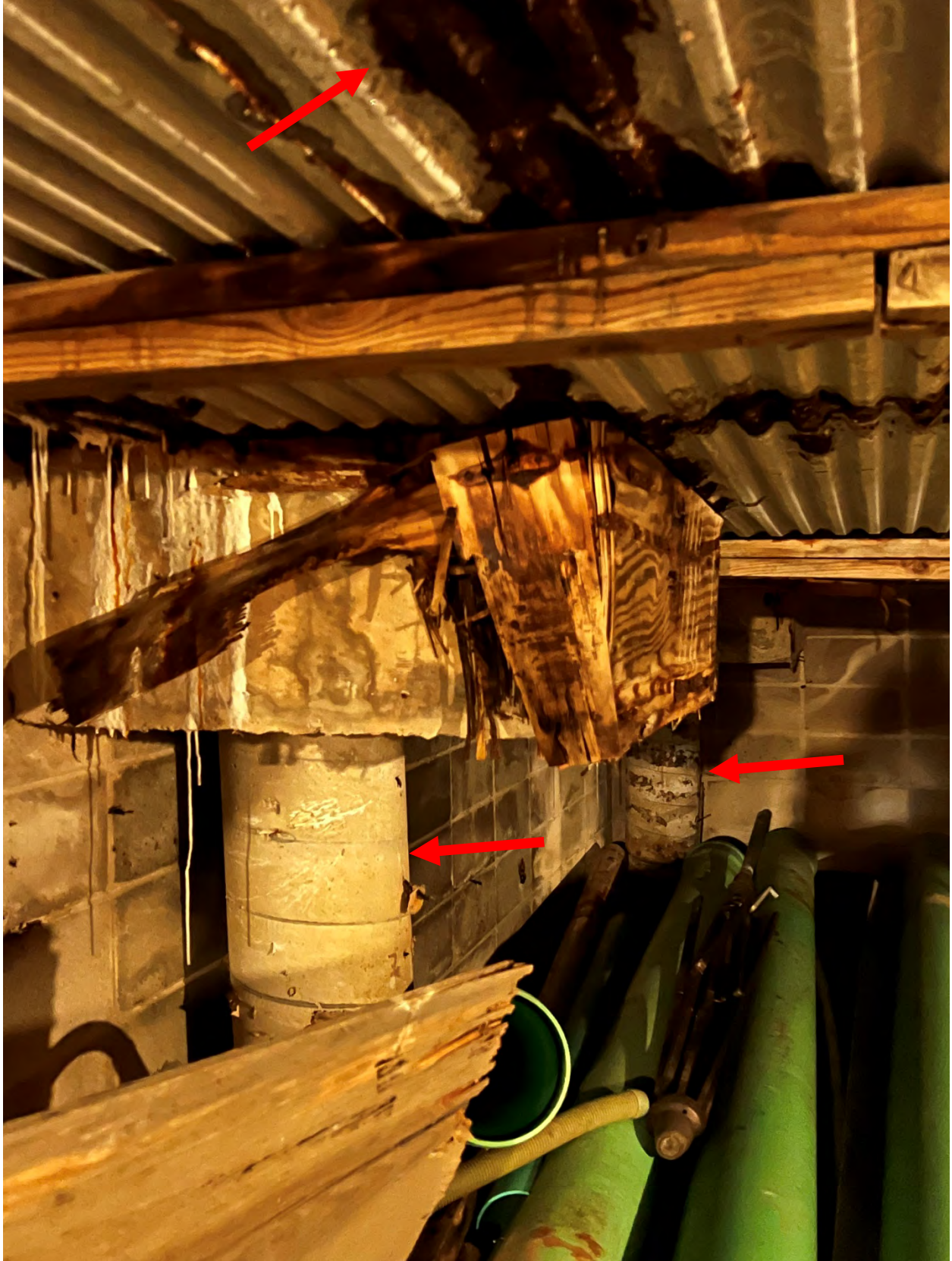
Photo #16 – View of typical deck corrosion at pool support structure. Piles visible in photo.
