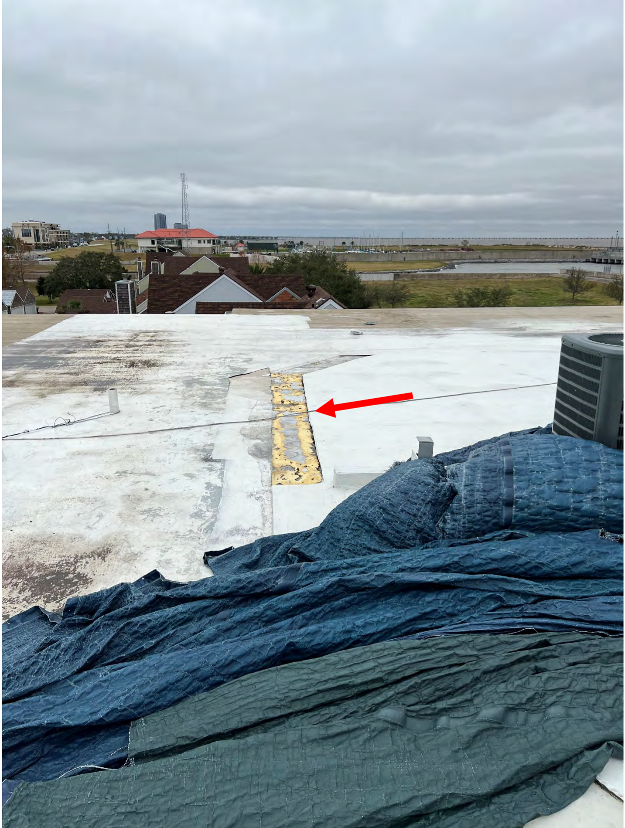
Photo #22 - View of missing roof membrane as a result of hurricane related wind damage
