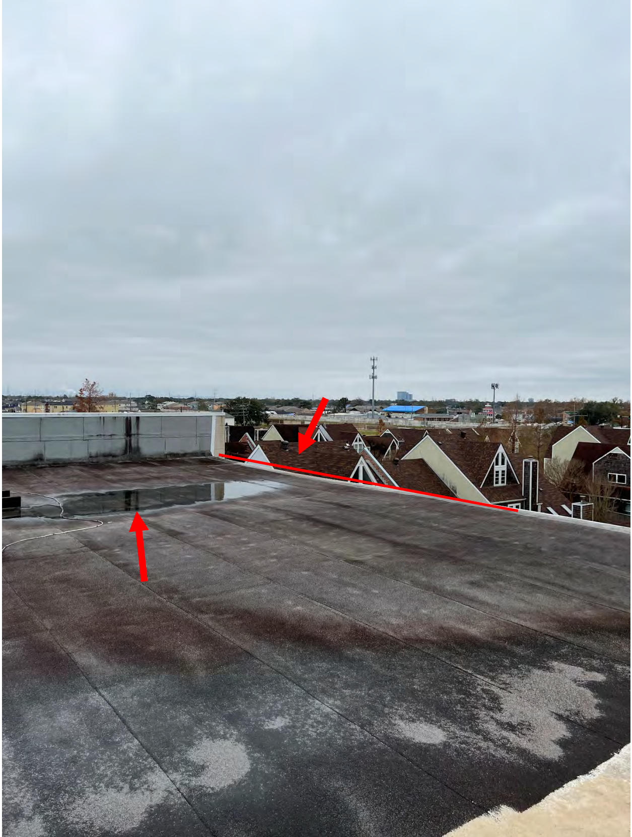
Photo #24 – View of noticeable sag at roof edge and concerning ponding in the near vicinity.
