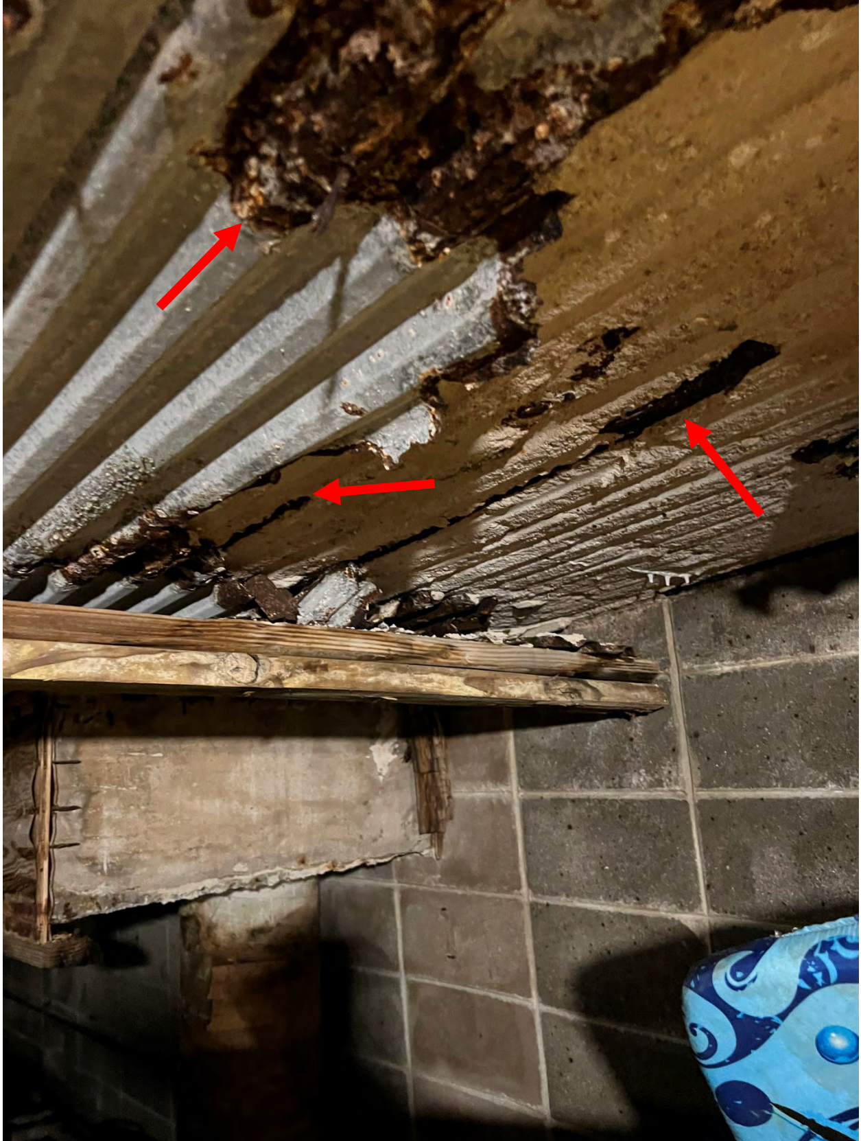
Photo #17 – View of exposed slab reinforcing and metal decking exhibiting severe corrosion.
