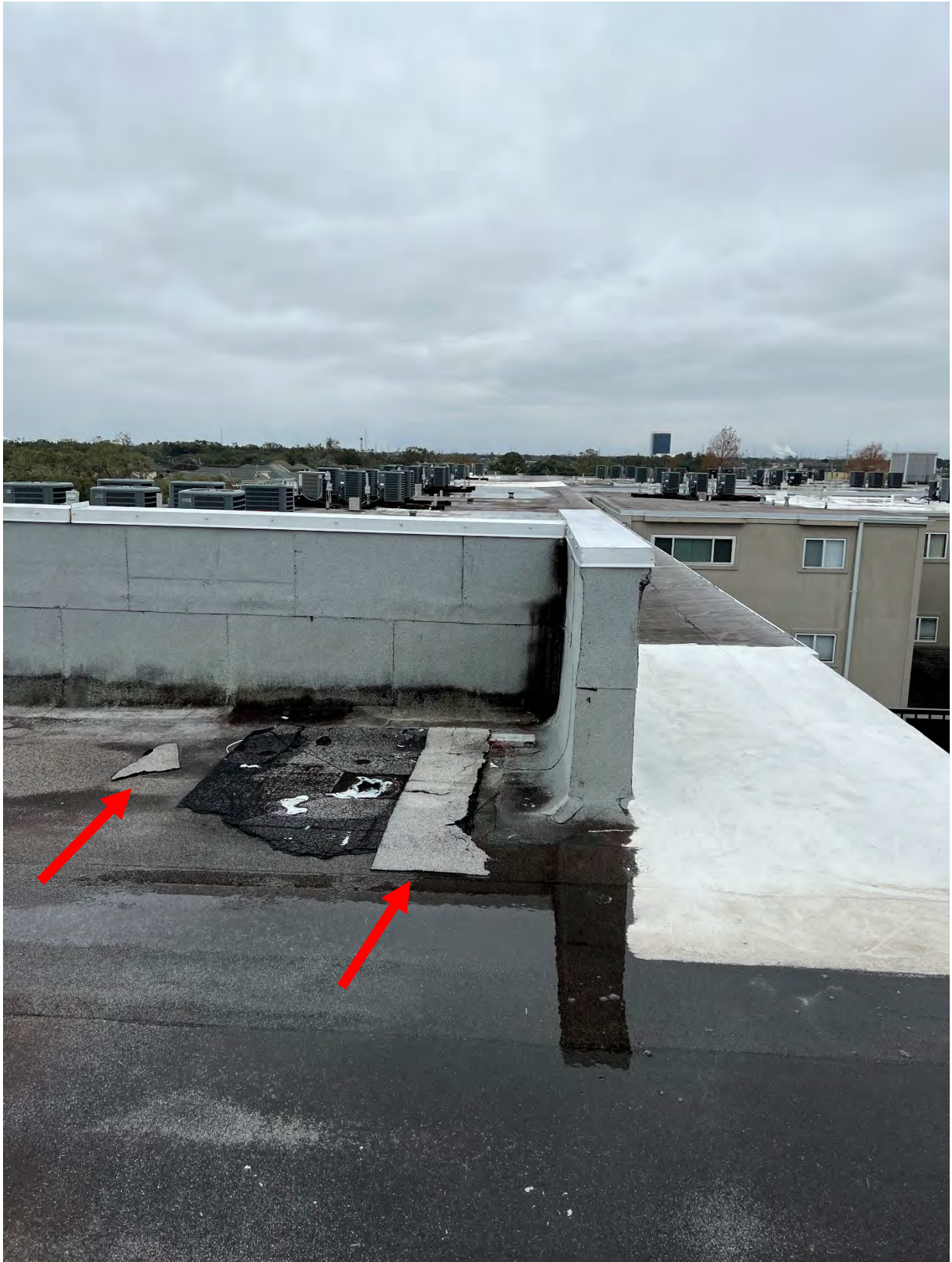
Photo #23 – View of roofing debris scattered as a result of hurricane related wind damage.
