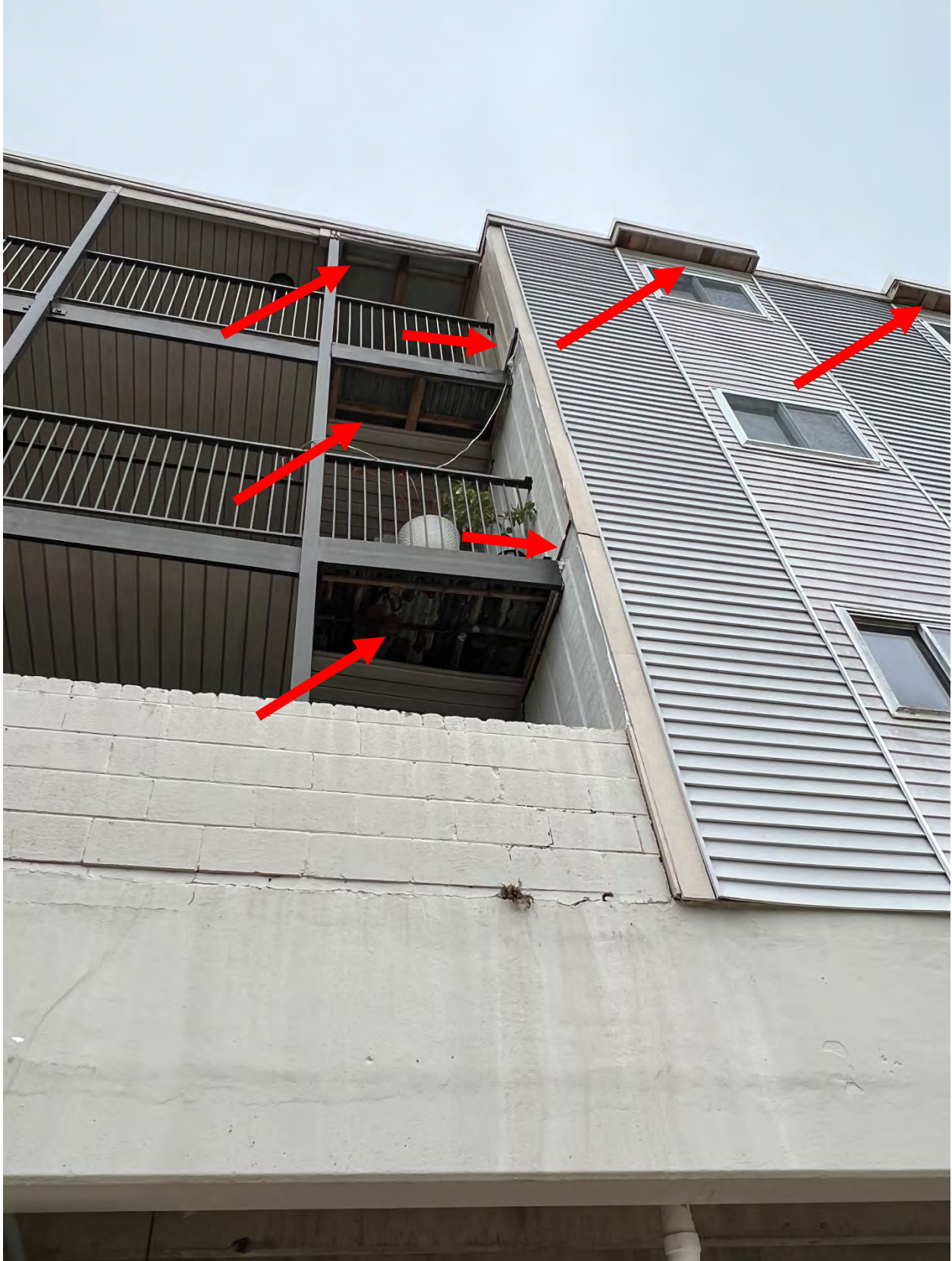
Photo #6 – View of wind related damages to corridor and roof soffits and exterior siding.
