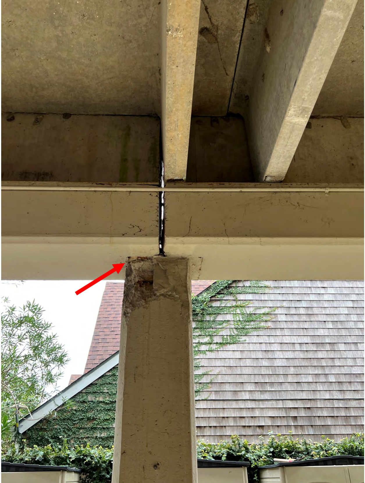
Photo #4 – View of typical top of column concrete spalling. Rusting of embed plate is visible.
