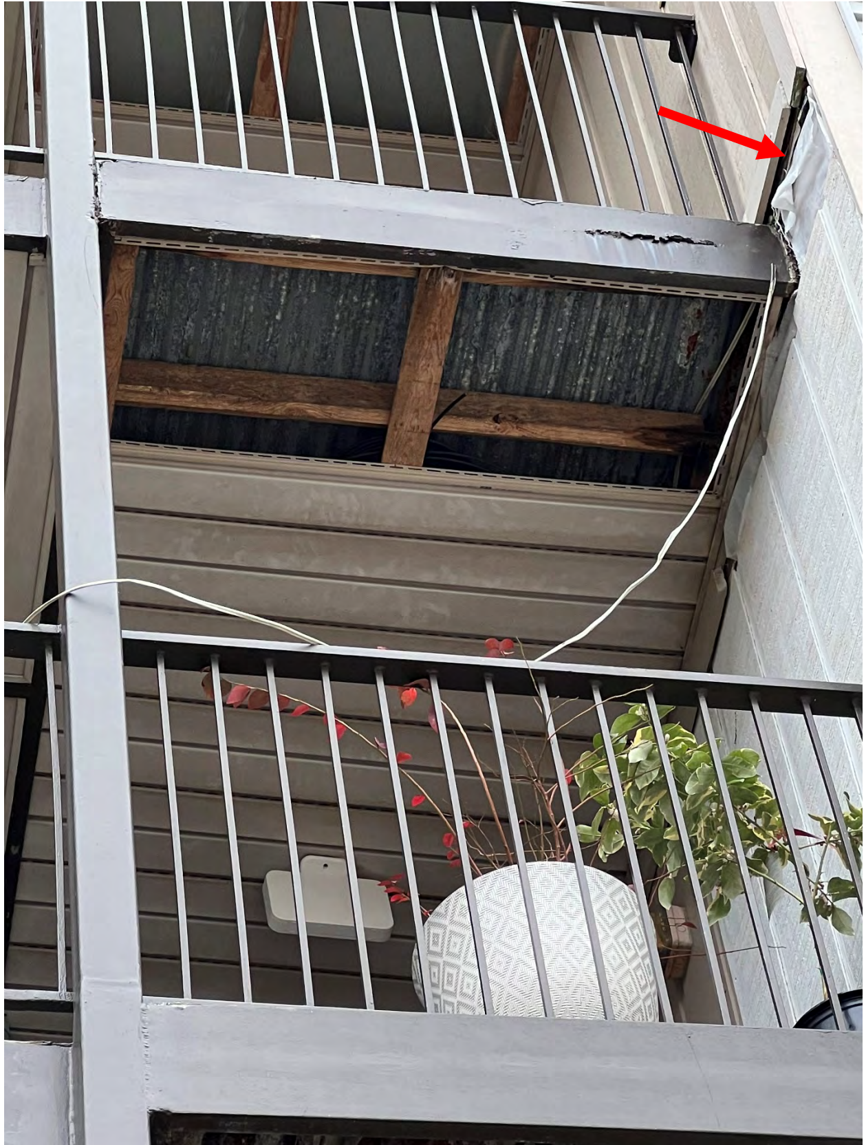
Photo #7 – Close up view of soffit and siding damage.
